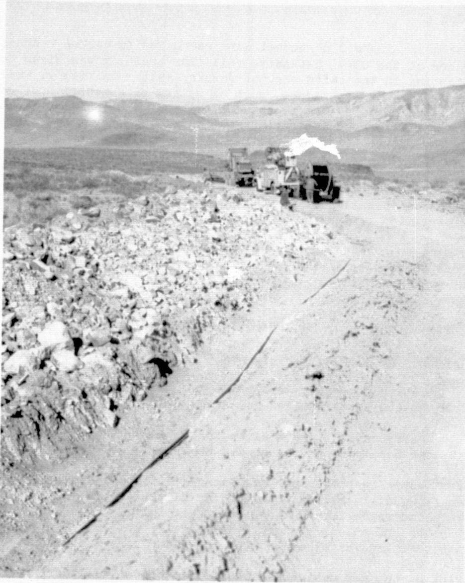
Fig. 42. Power and communication cable location
