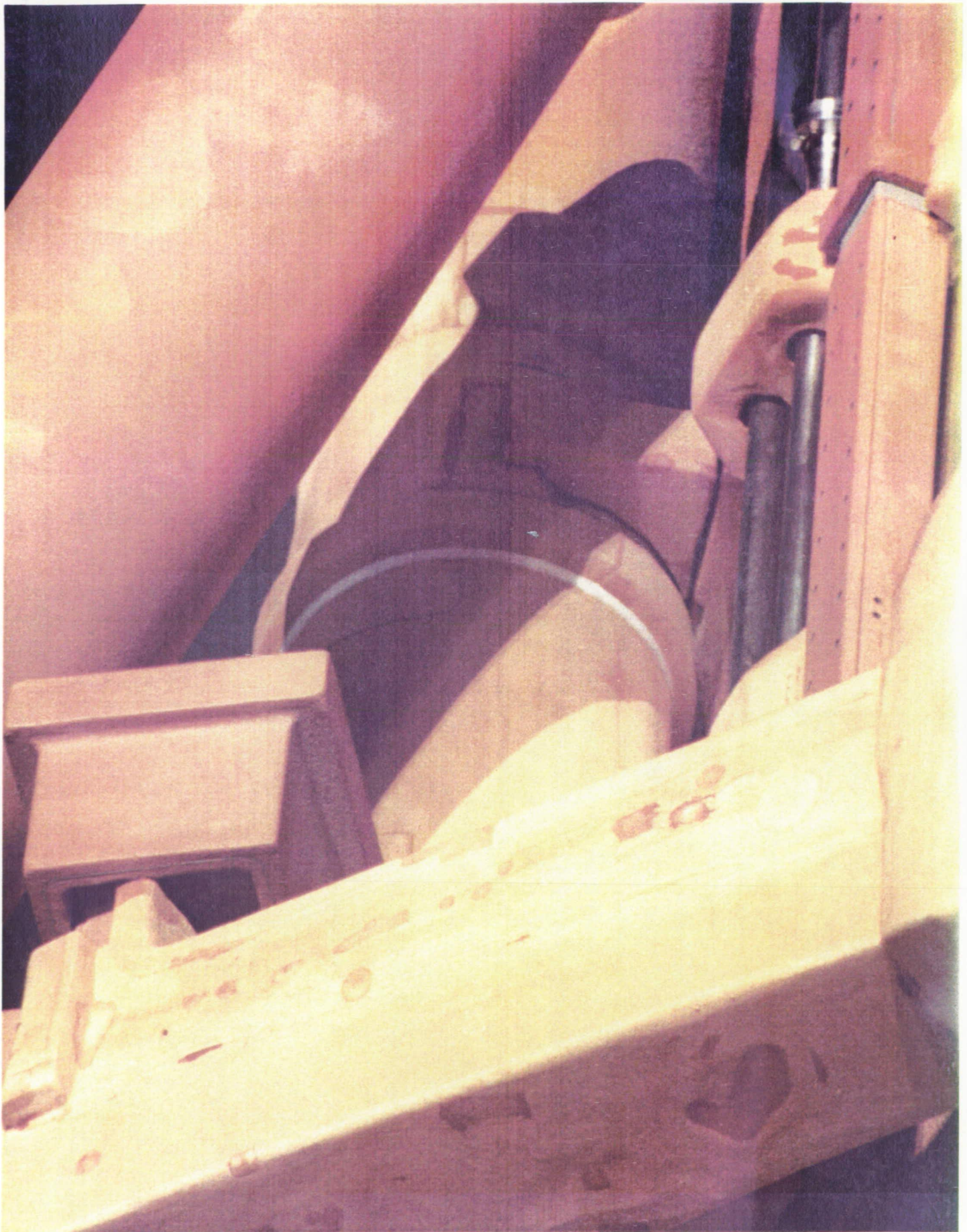
Typical ice/frost accumulation in the L02 feedline lower bellows and support brackets
