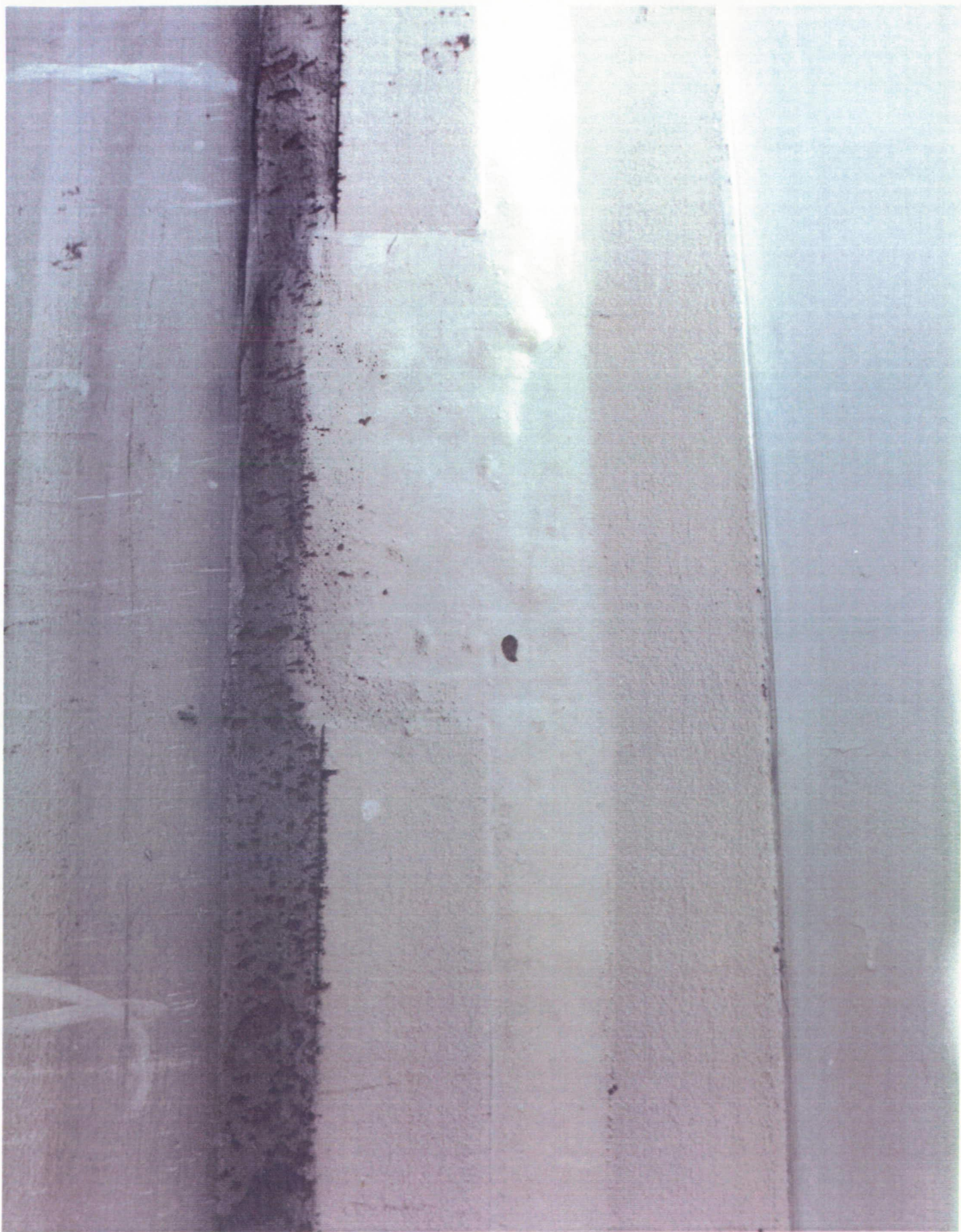
K5NA closeout blistered, or delaminated, in the center field joint
