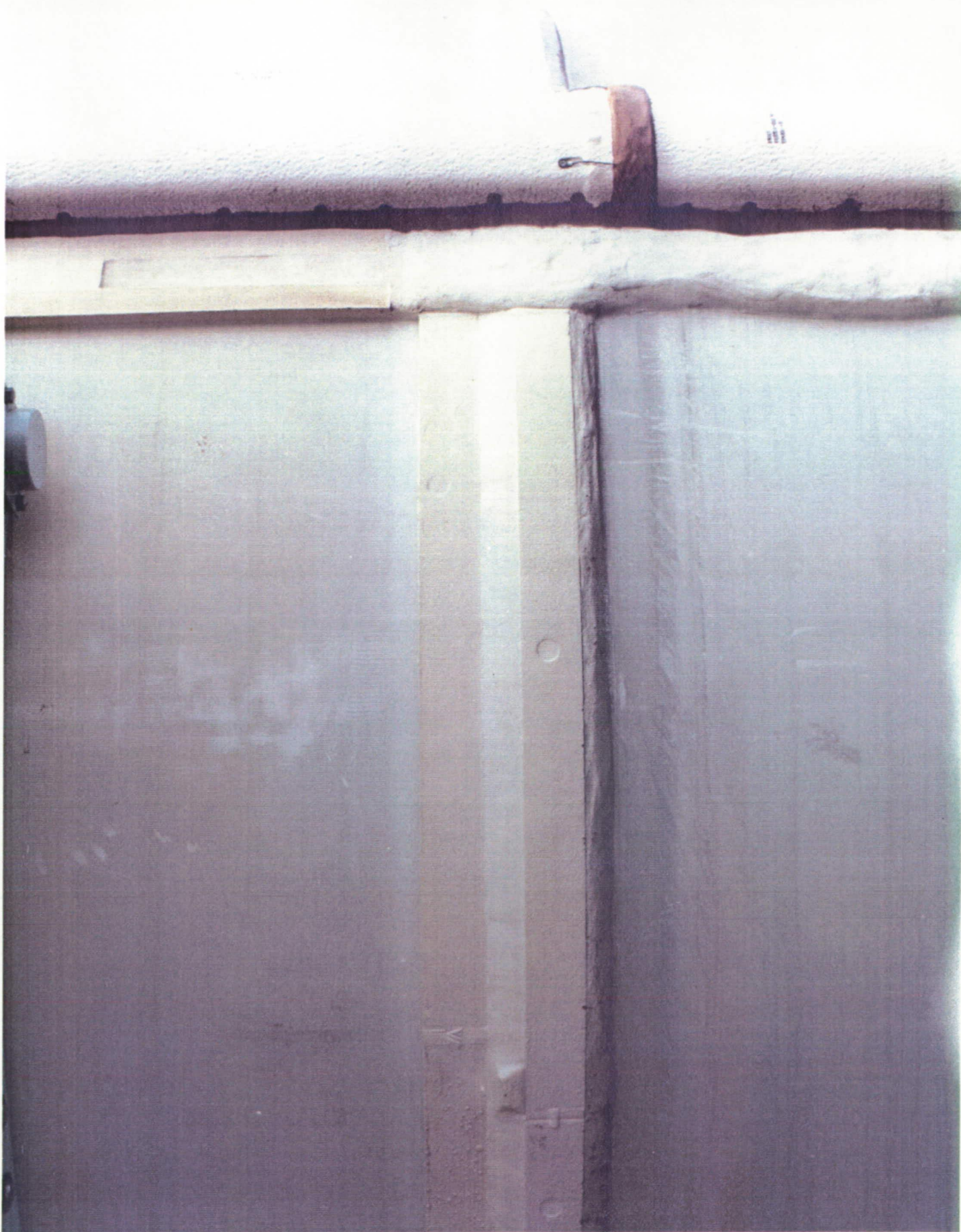
New Field Joint Protection System (FJPS) closeouts were in generally good condition
