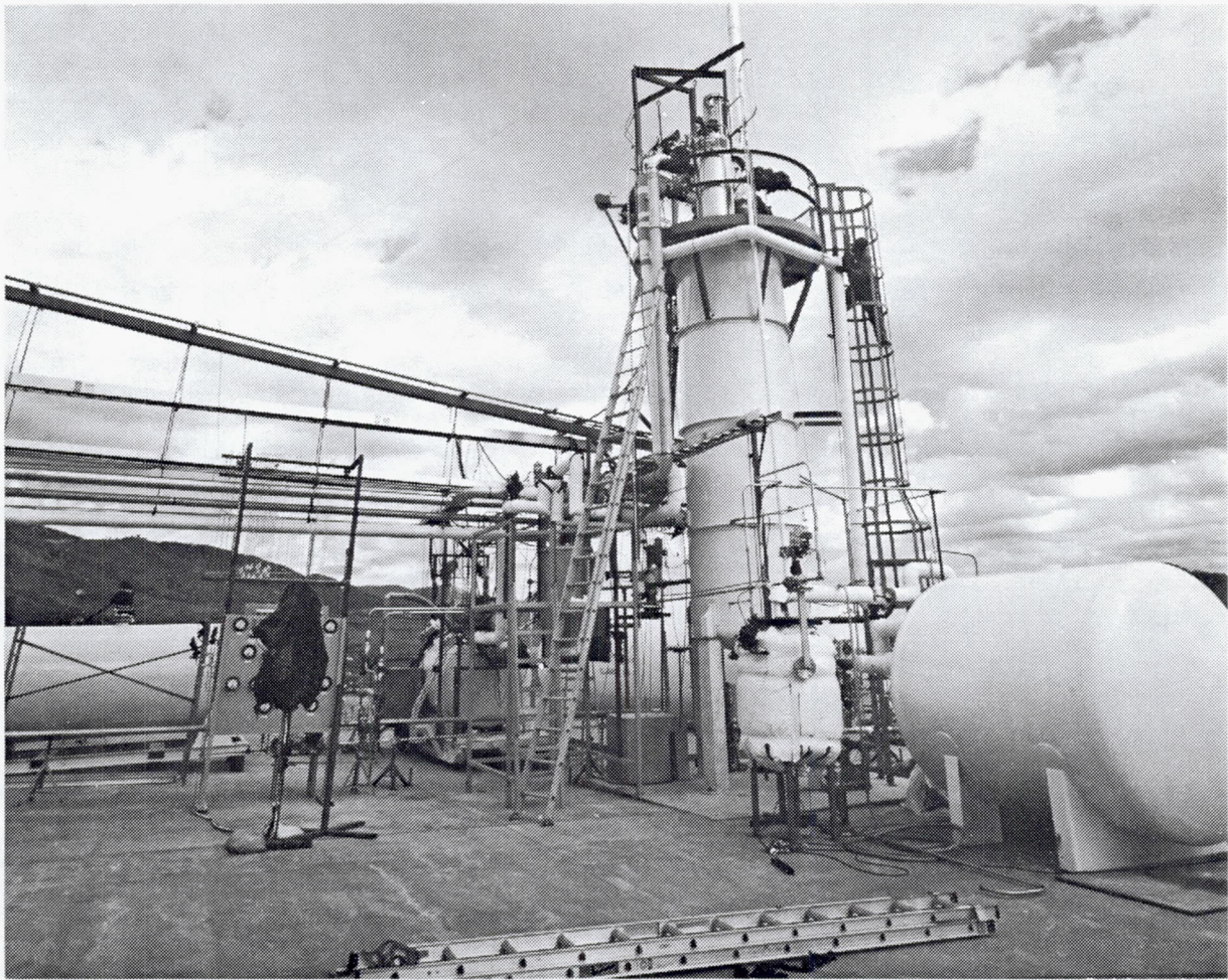
Figure 3-15. Pressurant Heat Exchangers and Slush Generator View
