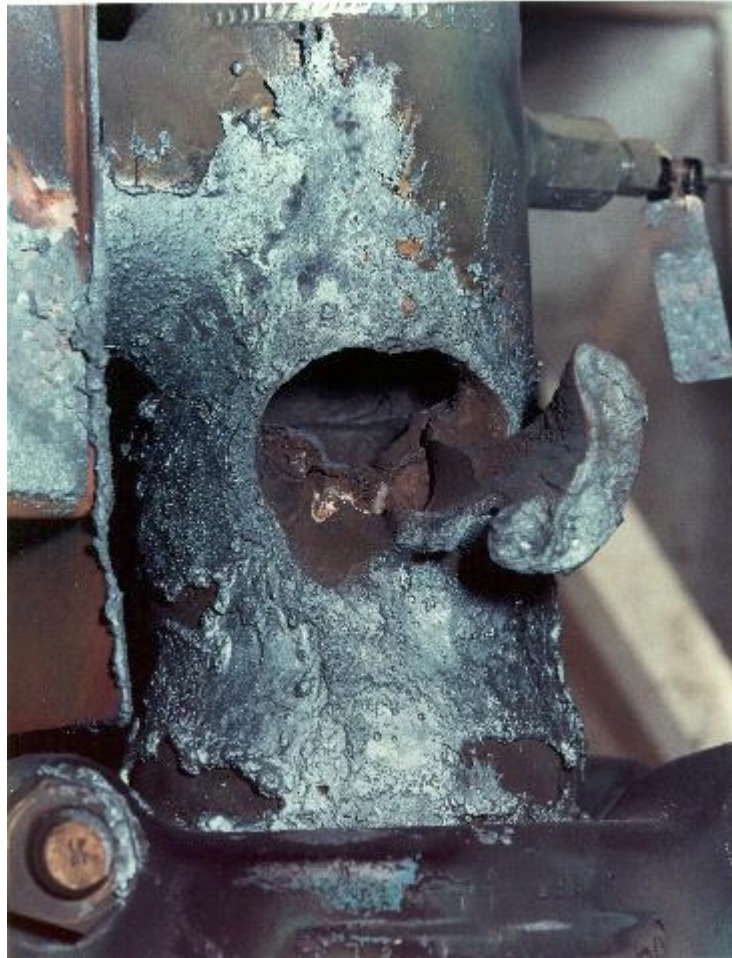
Figure 2 Burnthrough of First Test Apparatus, Right Vent Port
