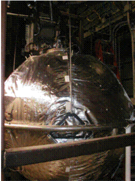
Figure 3.—14 m dia spherical tank shown with insulation assembled.
