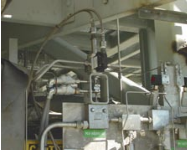
The high-pressure gaseous oxygen panel which feeds the ignition system for a rocket engine combustion device, located at ground level on the E-I Test Facility, Cell 3. The valve identified as PCV-10A2892-GO is operated by means of the high-performance actuator developed as a part of the Dual-Use Cooperative Agreement with BAFCO, Inc.
