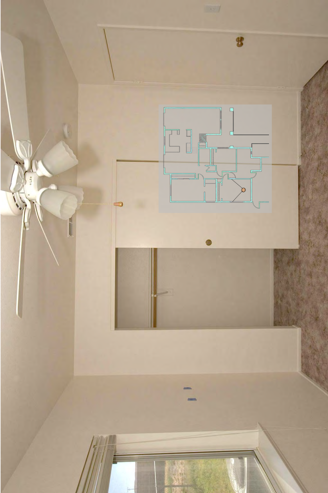
Garage bedroom, west wall. Viewpoint relative to floor plan is illustrated in the inset.
