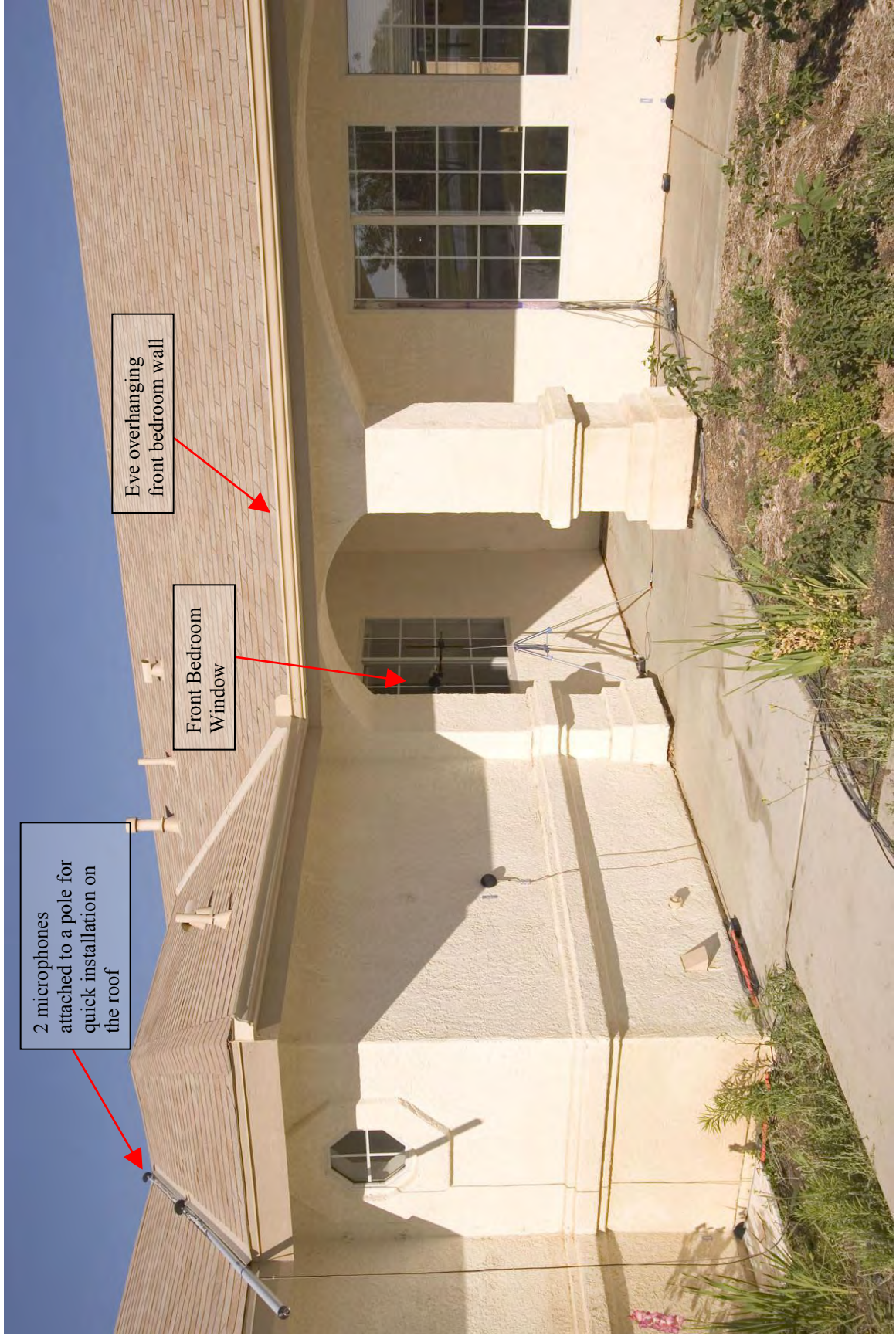
View of the front of the house at 52 Blackbird Street looking south west at the exterior walls of the front bedroom and main living area.
