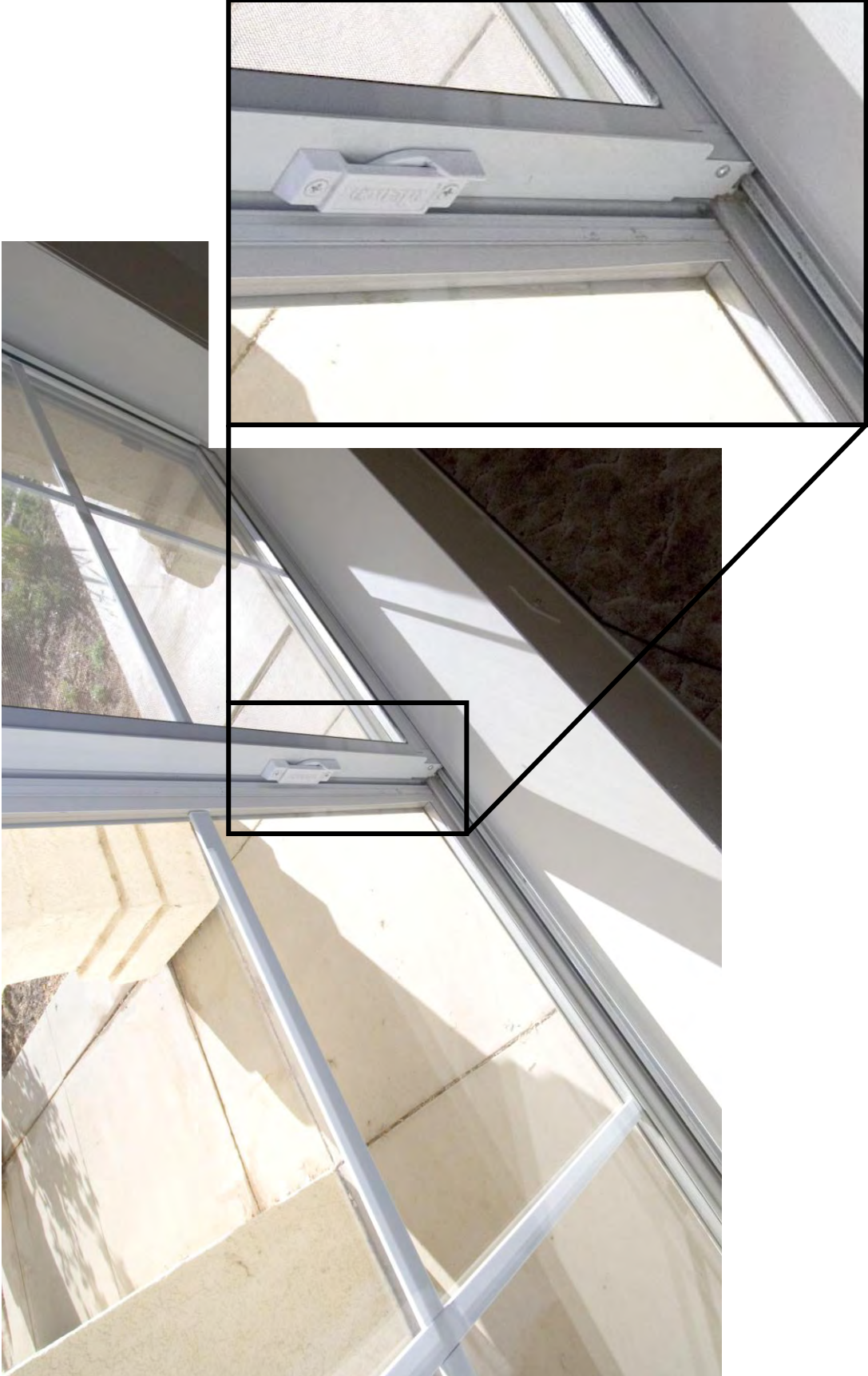
Figure 2.14: Detailed photograph of both the sliding and fixed portion of the front bedroom window.
