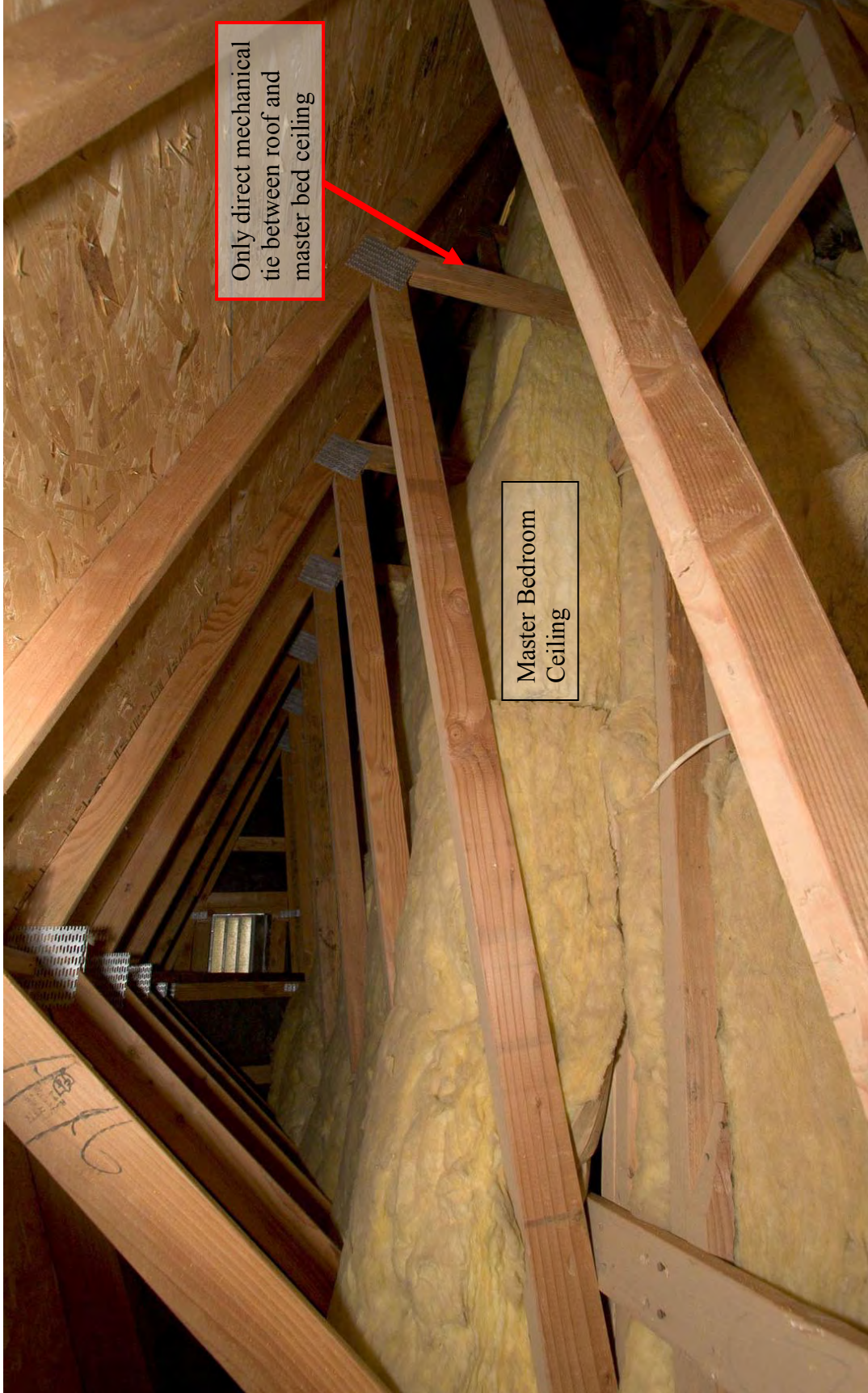
Figure 2.17: View of the attic above the main living area and master bedroom, looking south, over the master bedroom.
