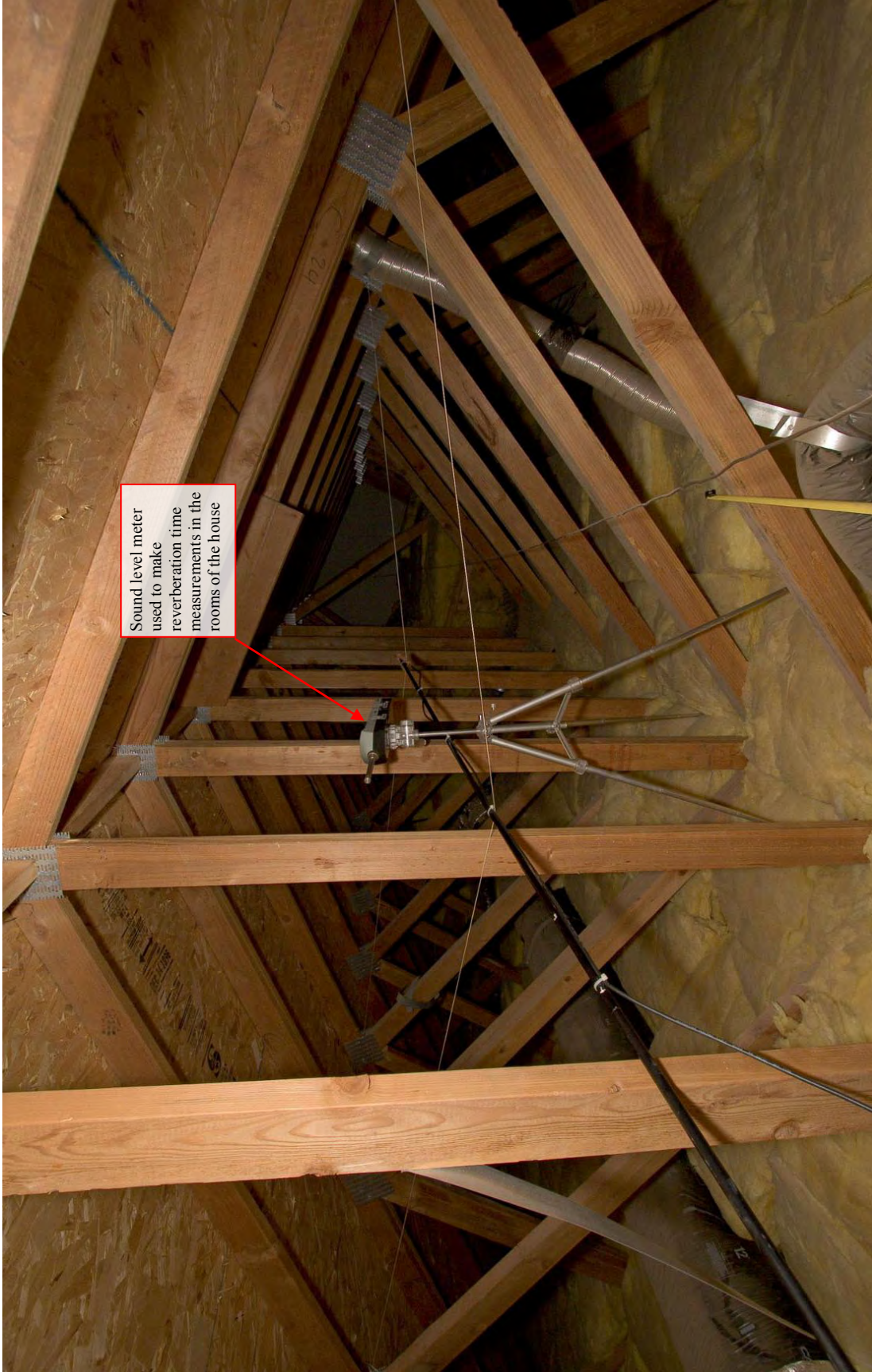
Figure 5.2: Photograph of the sound level meter in the attic for reverberation time measurements.
