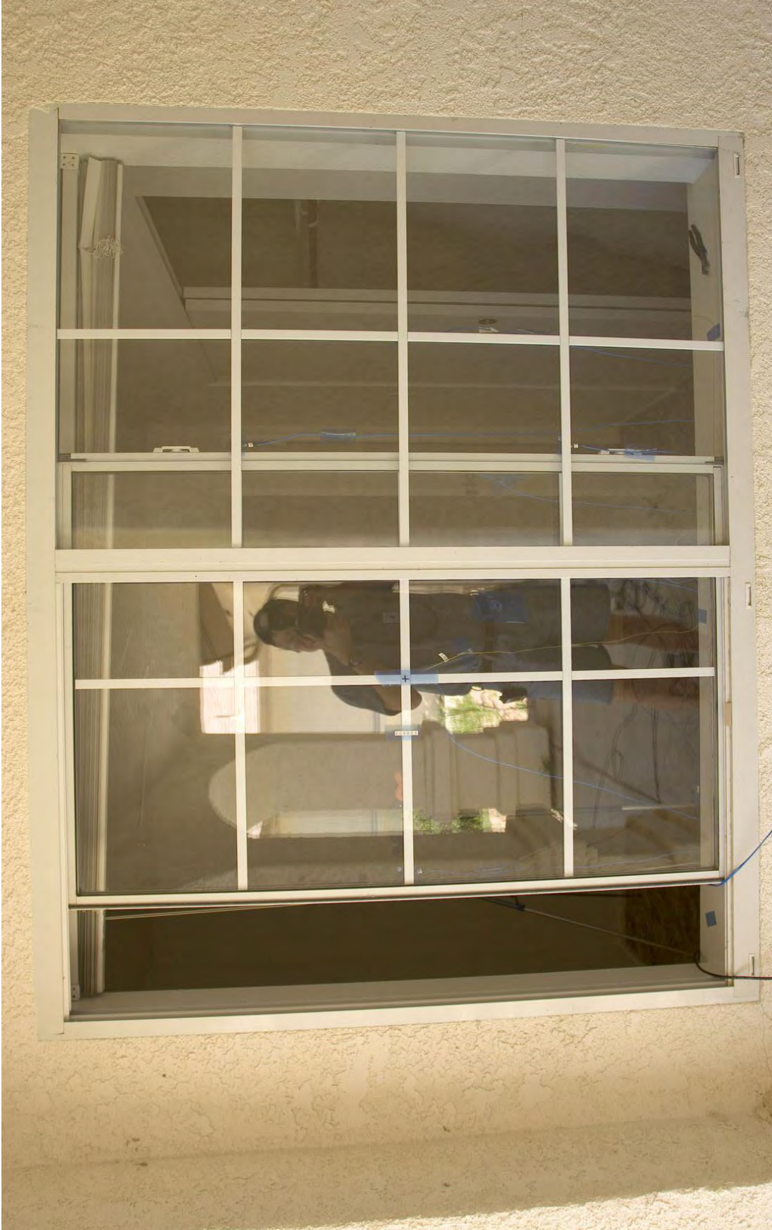
Figure 3.16: Front bedroom window was opened approximately 6-inches for the tests on July 18 th , 2007.
