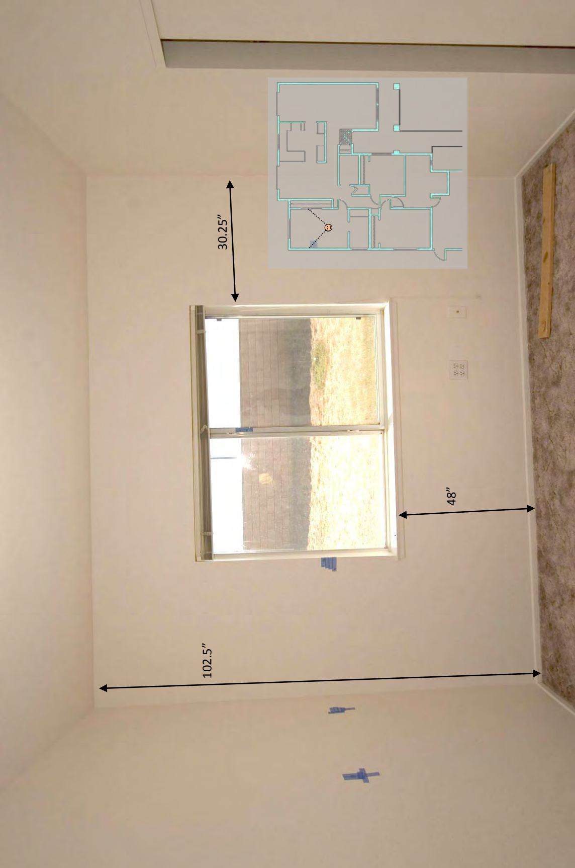
Master bedroom, west wall. Viewpoint relative to floor plan is illustrated in the inset.
