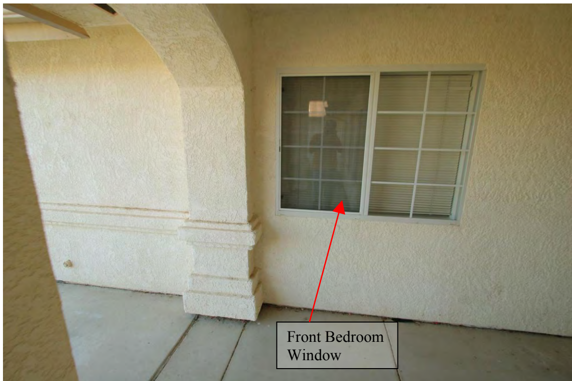
Figure 2.23: View of the front of the house looking south at the exterior wall of the front bedroom.
