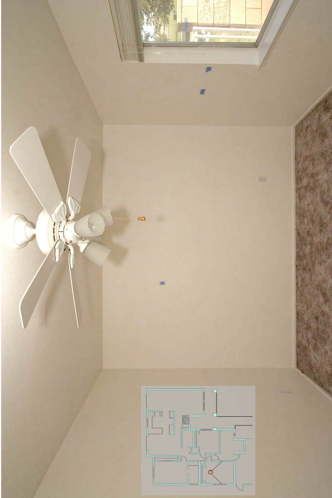
Garage bedroom, east wall. Viewpoint relative to floor plan is illustrated in the inset.
