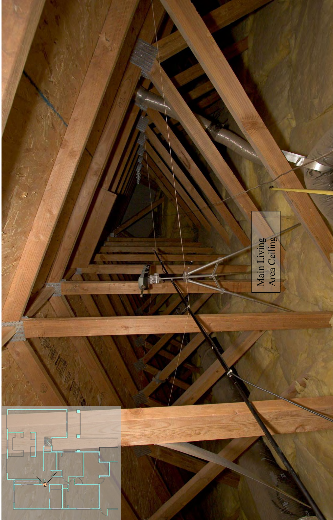
View of the attic above the main living area and master bedroom, looking north, over the main living area. Viewpoint relative to floor plan is illustrated in the inset.
