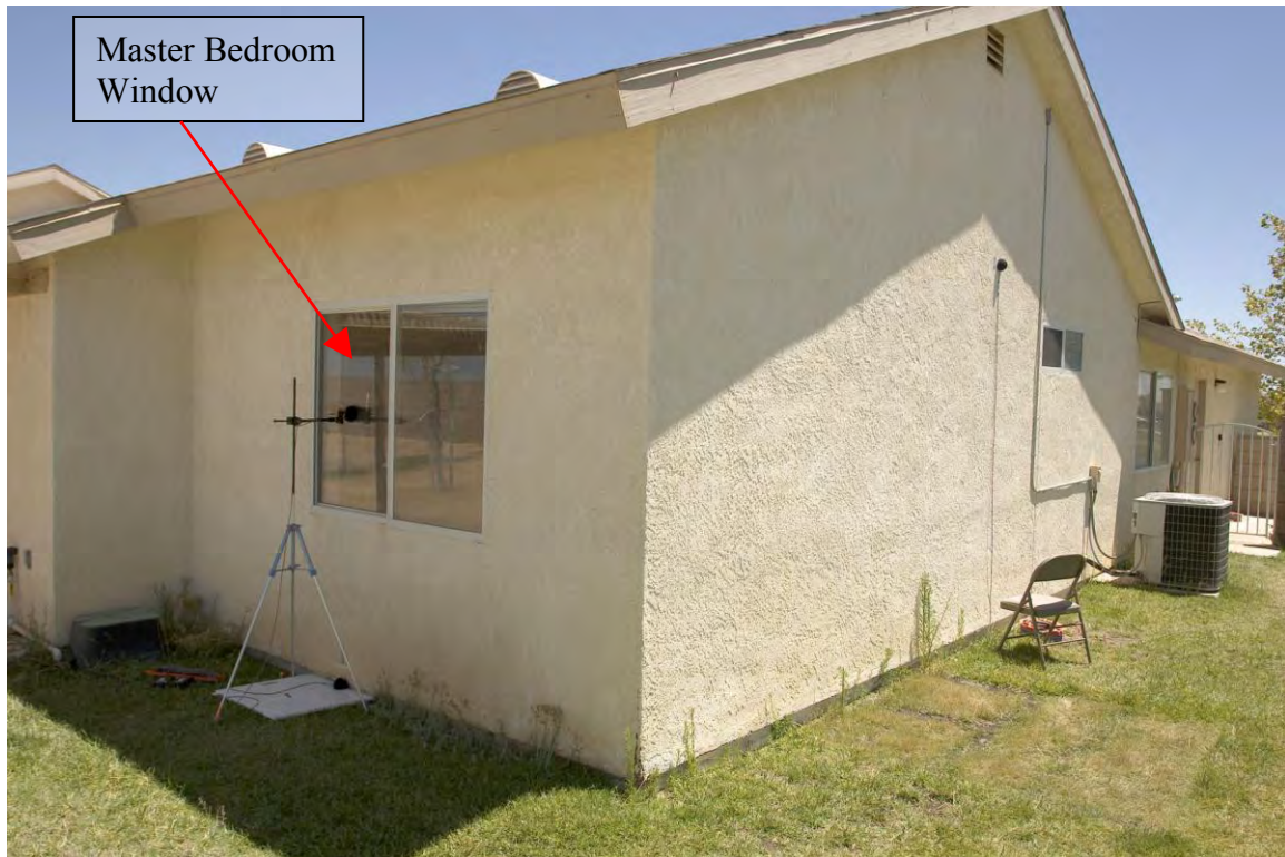
Figure 2.26: View of the side of the house looking southeast at exterior wall of the master bedroom.
