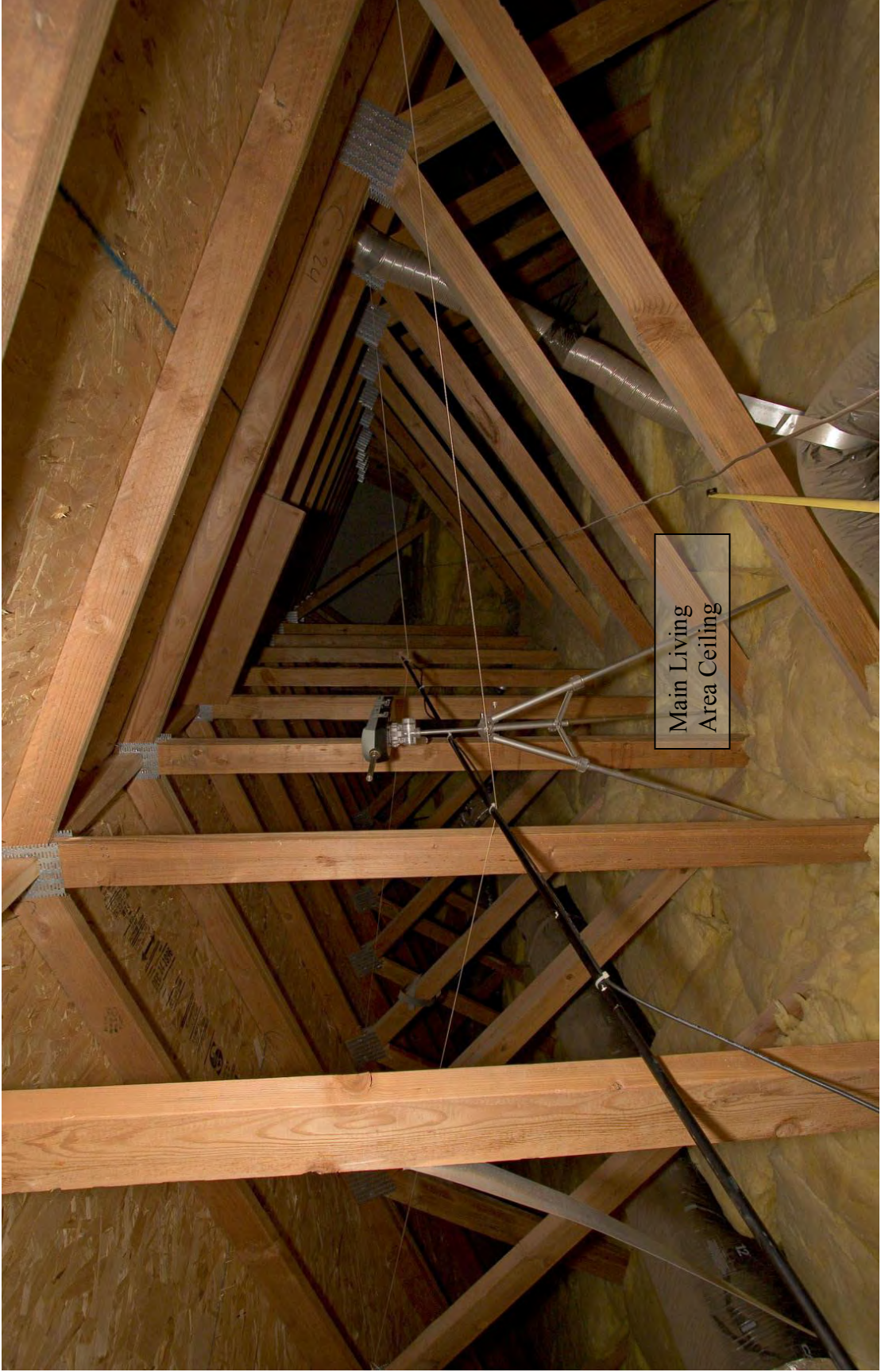
Figure 2.18: View of the attic above the main living area and master bedroom, looking north, over the main living area.
