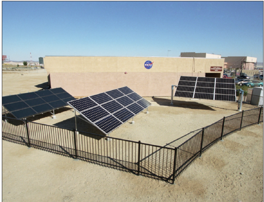
Figure 1. This Solar-Panel Array Demonstration Site at NASA's Dryden Flight Research Center is a facility for testing the most advanced solar photovoltaic cells commercially available for terrestrial applications. NASA photo by Tom Tschida.
