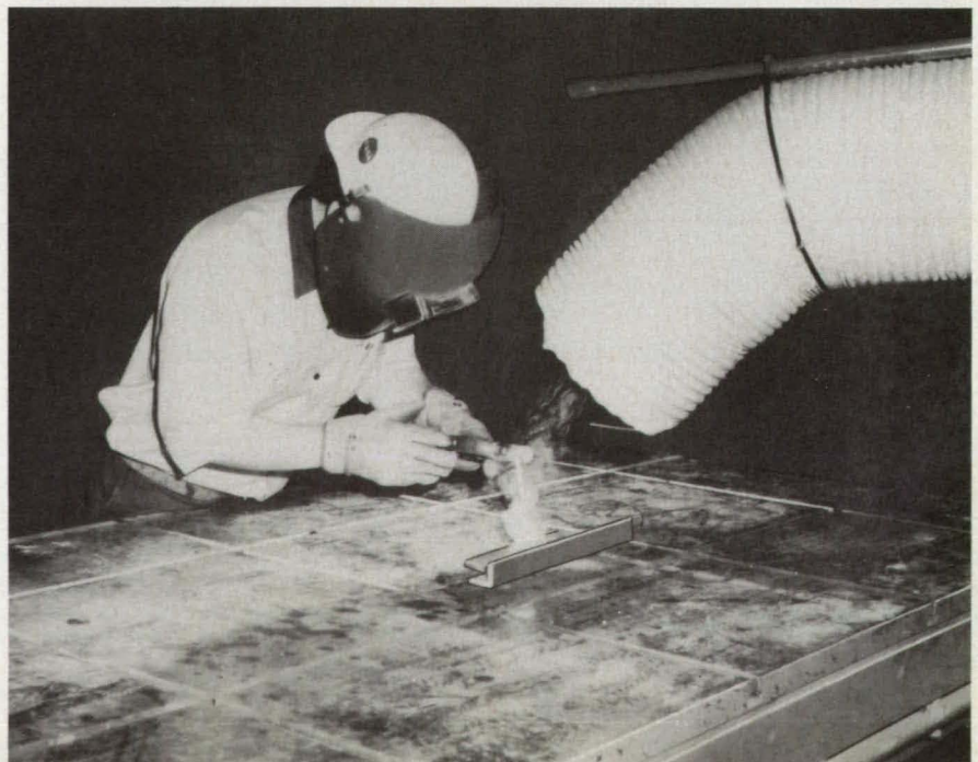
Figure 1. The Exhaust Duct Scoops Up welding fumes at one end and passes them to the exhaust system at the other.
