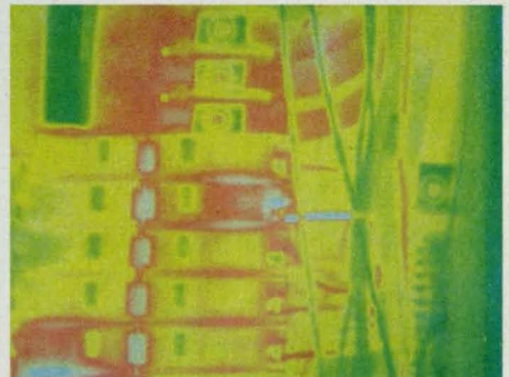
A thermal video system can show you a hot component and, with hard-disk image storage and retrieval, allow on-the-spot trend analysis.
