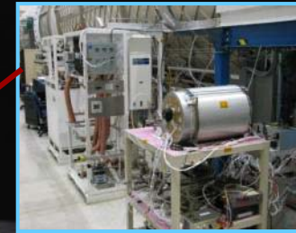
Exploration Water Recovery System (EWRS)
