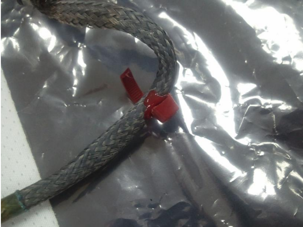
Figure D.53.—Wire harness for Heater 1: Note melted ty-rap.
