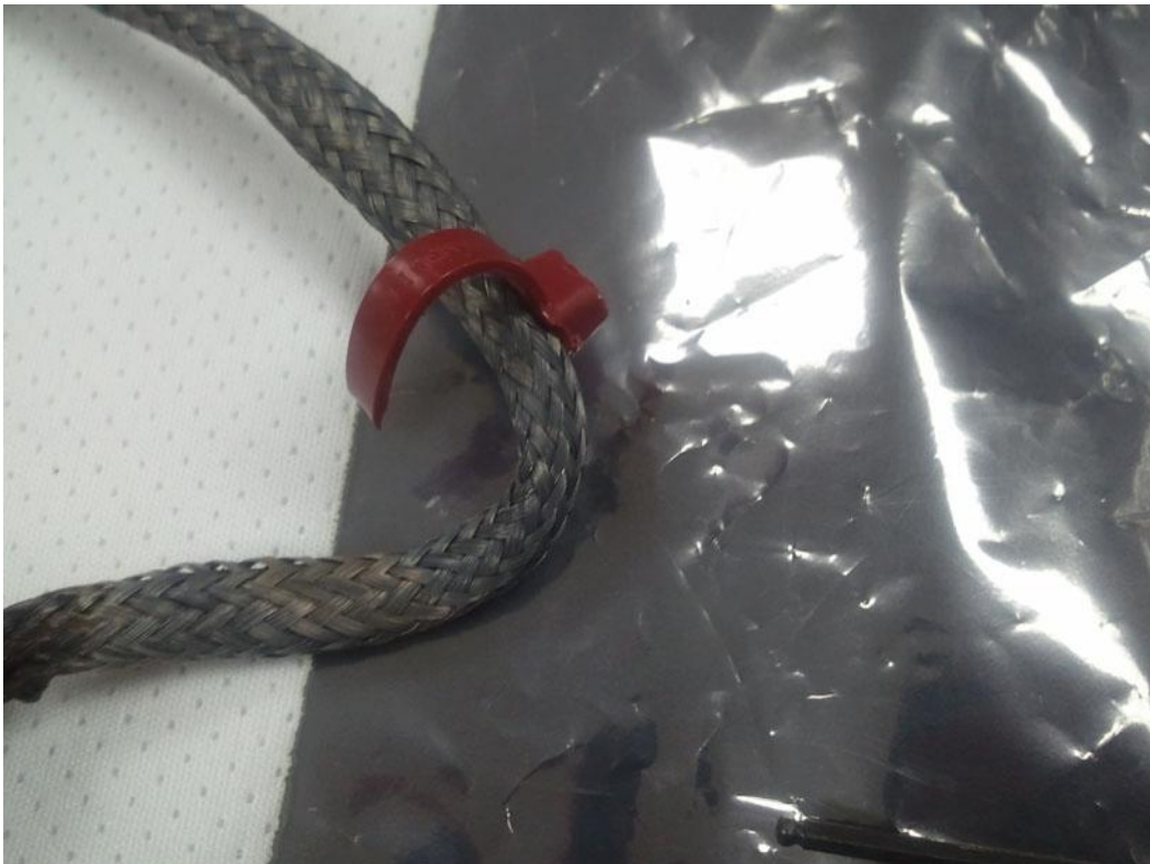
Figure D.50.—Wire harness for Heater 1: Note melted ty-rap.
