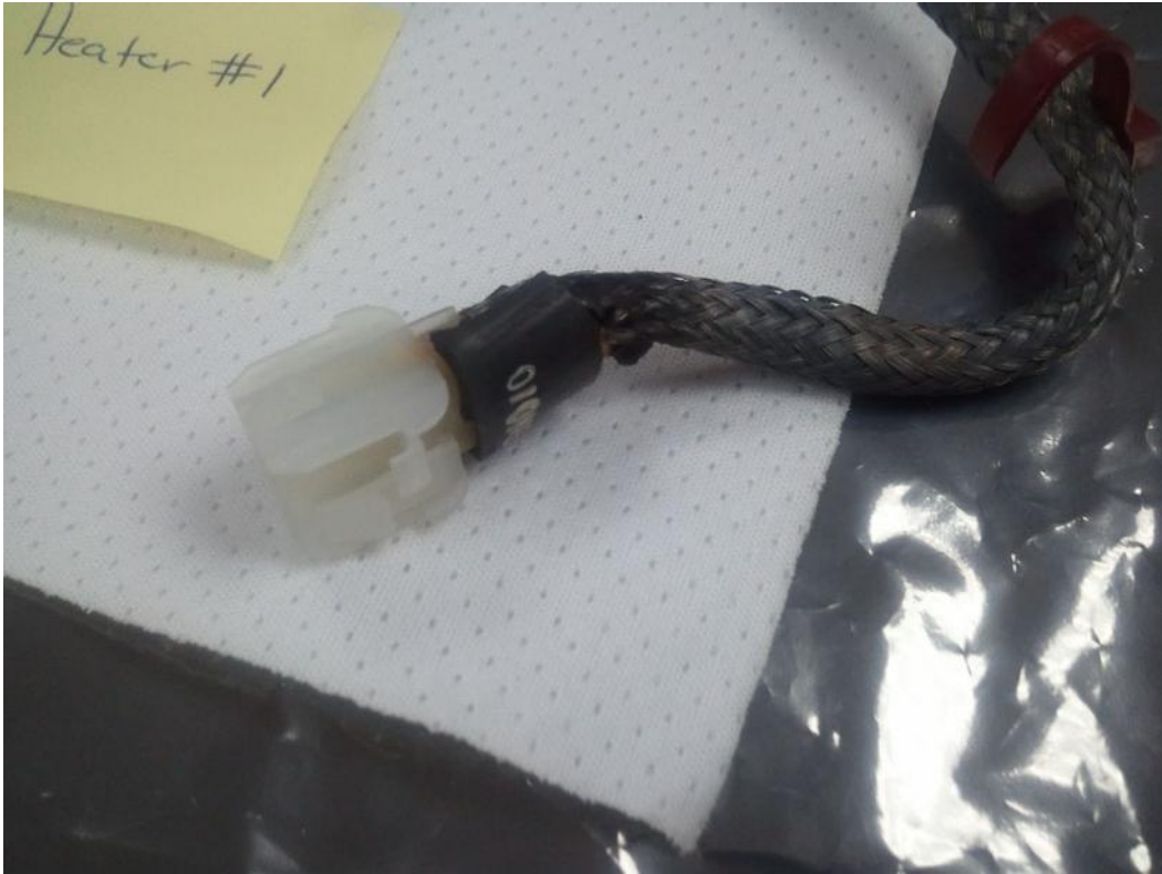
Figure D.49.—Heater 1 Molex connector, note discoloration on wire braid.
