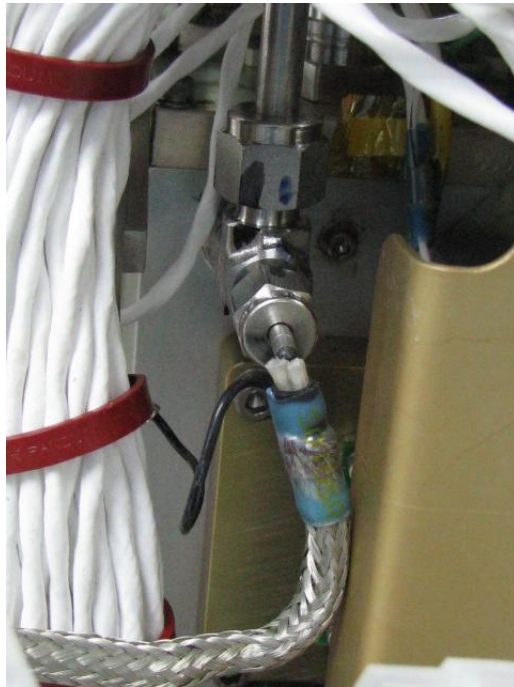
Figure D.61.—Heater 2 connection into TC.
