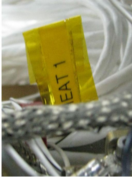
Figure D.1.—Heater 1 power cable.
