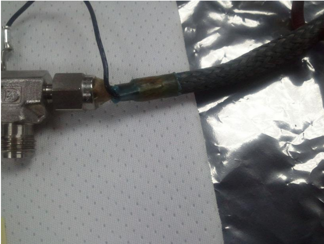
Figure D.55.—Heater 1 connection into TC.
