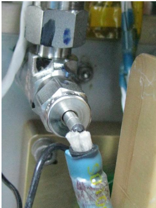
Figure D.59.—Heater 2 connection into TC.
