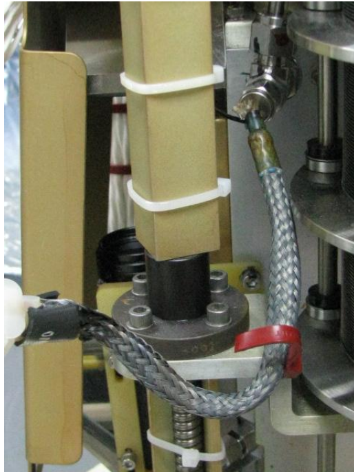
Figure D.9.—Heater 1 power cable, note discoloration on wire braid by Molex connector and melted ty-rap.
