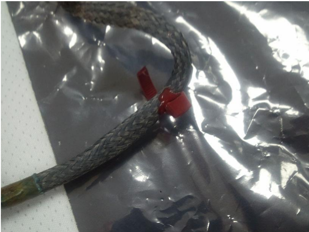
Figure D.52.—Wire harness for Heater 1: Note melted ty-rap.
