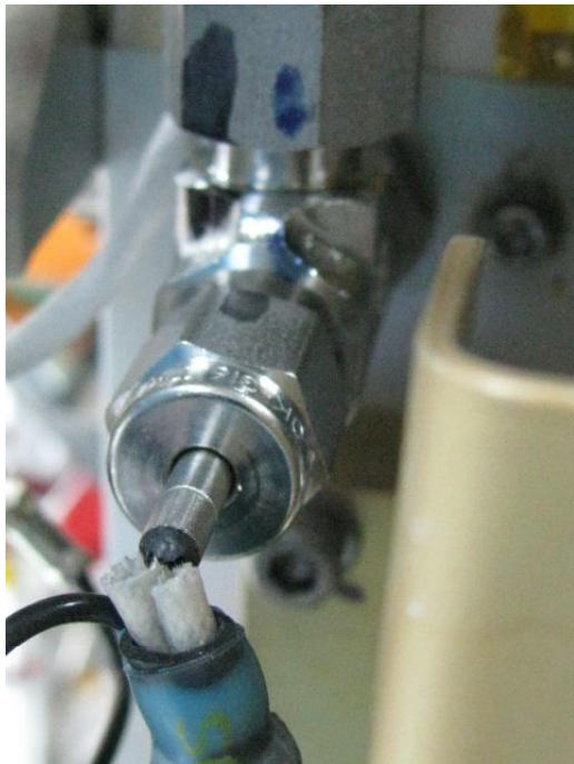
Figure D.60.—Heater 2 connection into TC.
