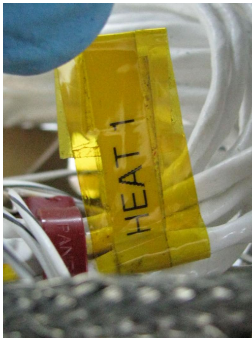
Figure D.2.—Heater 1 power cable.
