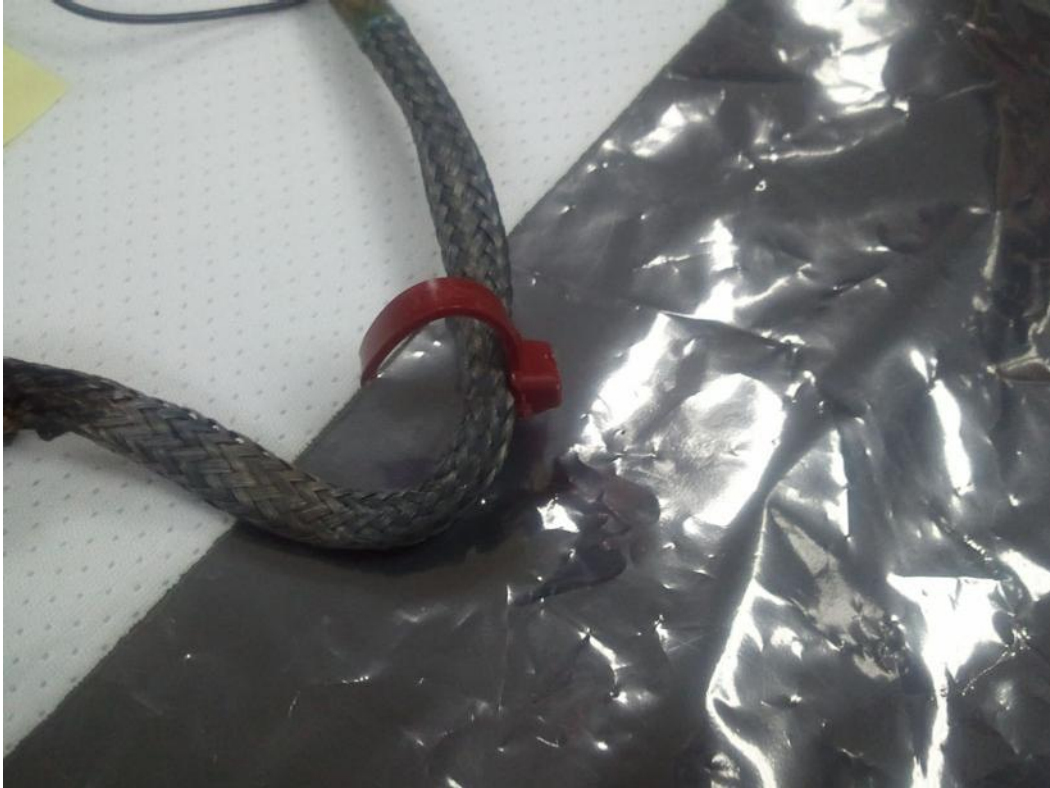
Figure D.51.—Wire harness for Heater 1: Note melted ty-rap.
