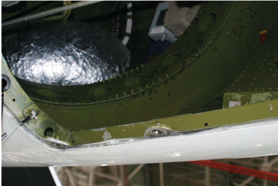
Figure 6.1-12. Falcon 20 Visually Inspected Fuselage Frame Showing Greasy Residue
