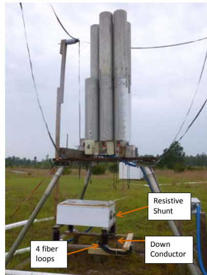
Fig. 13. Four loops of fiber optic current sensor installed under the rocket launch tubes.
