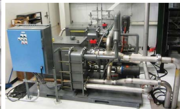
New Cooling Water System now provides 2 separate systems that cool induction coil and power feedthrough, induction heater and H 2 N 2 mixer respectively
