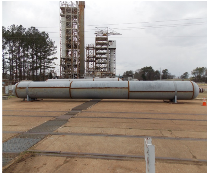
Figure 7.1.2.3-1. MSFC Vessel V0256 with Welds Stripped for Inspection (A225 head material; MLP 1143 shell material)
