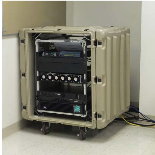
Figure 3. - Transportable ground station installed at Ohio University Airport
