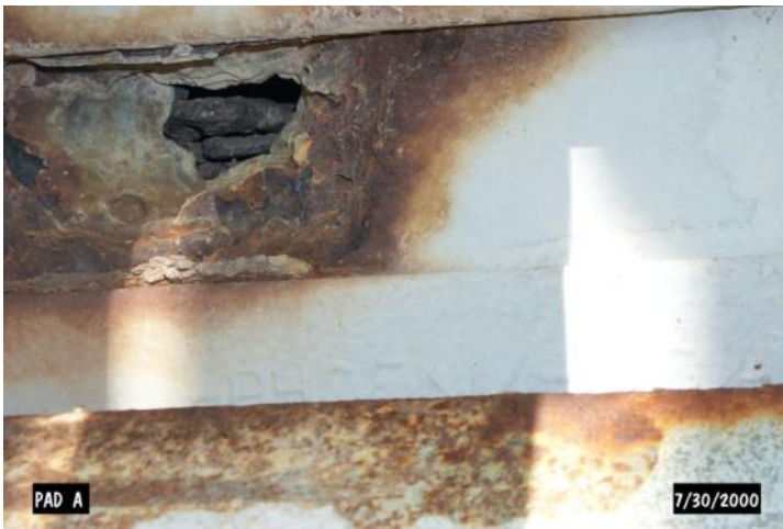
KSC Launch tower structural steel corrosion
