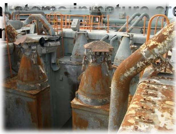
KSC Launch Pad Corrosion (after a Space Shuttle launch)
