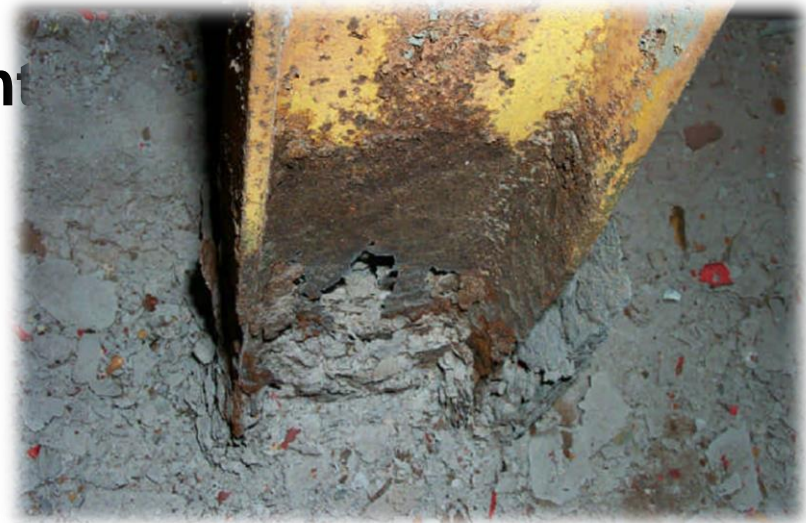
KSC Crawler/Transporter Structural Steel Corrosion
