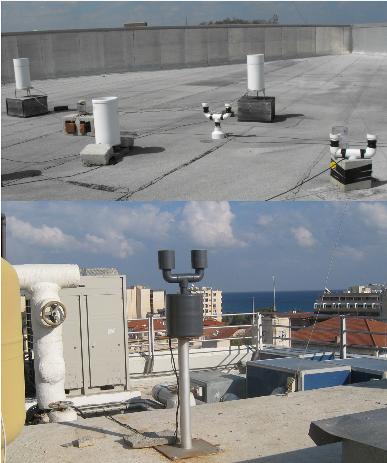
Fig. 1. (Color online) Top: Roof of UCF Engineering Building, showing three tipping bucket rain gauges (white cylinders) and three disdrometers: Joss disdrometer on left, and two UCF-DHD disdrometers in center and far right. Bottom: CUT-DHD on the roof of the Cyprus University of Technology.
