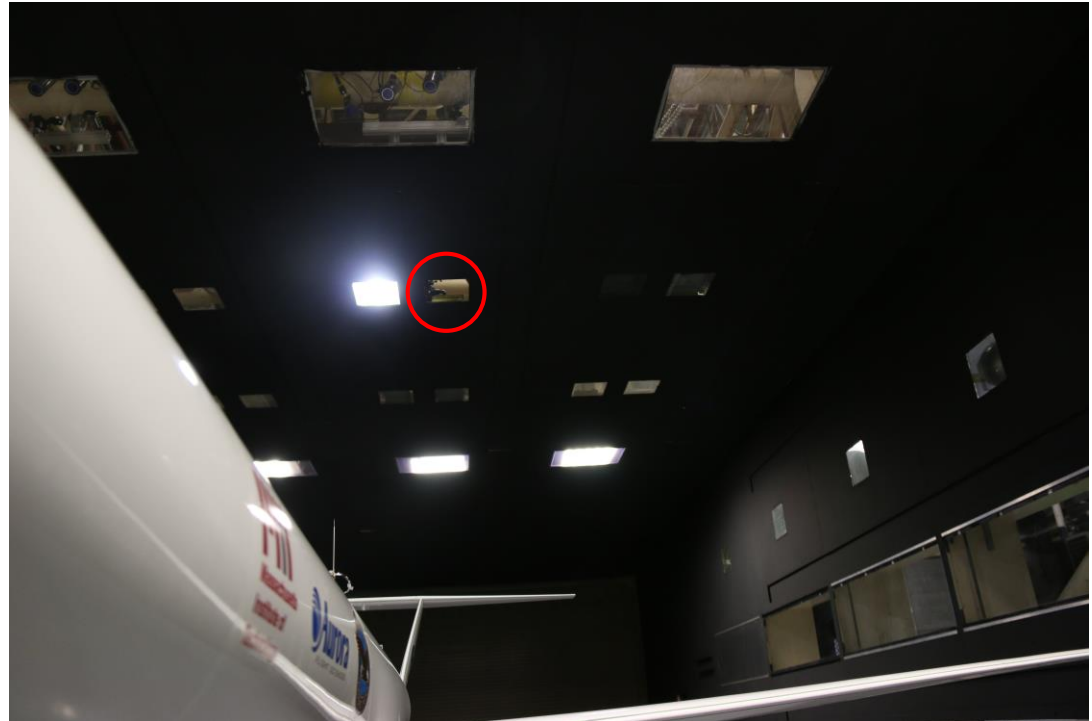
Bottom view, showing location of removed pane of glass in tunnel ceiling
