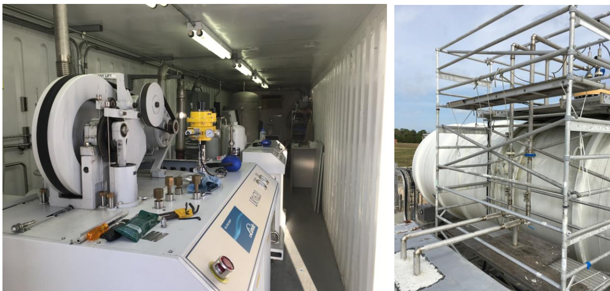
Figure 4: Refrigeration Container Showing the Refrigerator Module (foreground) and RSX Compressor (background) (left); GHe VJ Piping Interfaced to IRAS Tank (right)
