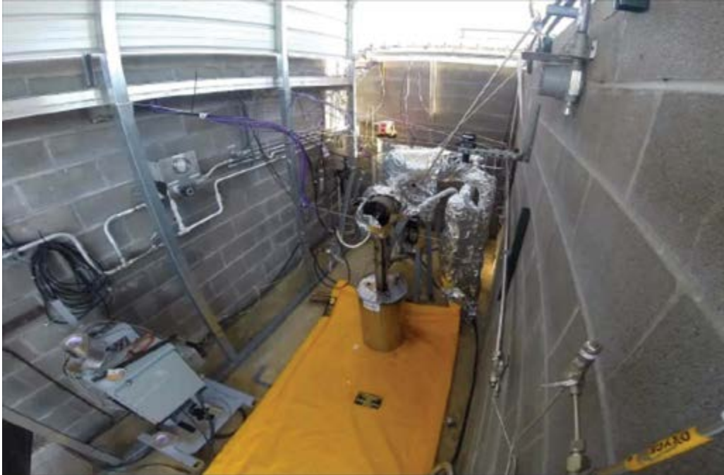
Figure 1: F-16 gas generator installed at MSFC Component Development Area Test Cell.
