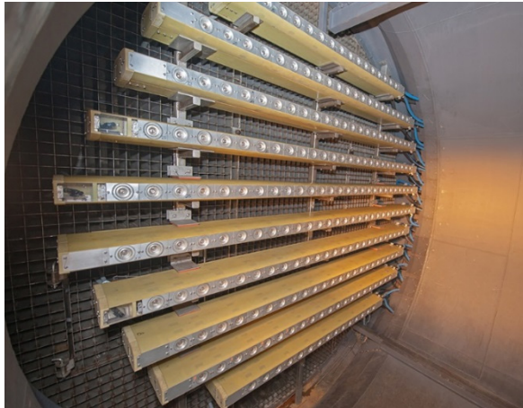
Figure 2.—PSL-3 spray bar system.
