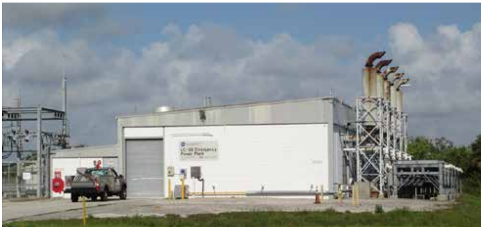
C5 Emergency Power Station - Oxidation catalysts were installed at the exhaust side of the engines in 2014 reducing CO emissions by \geq to 70%.
