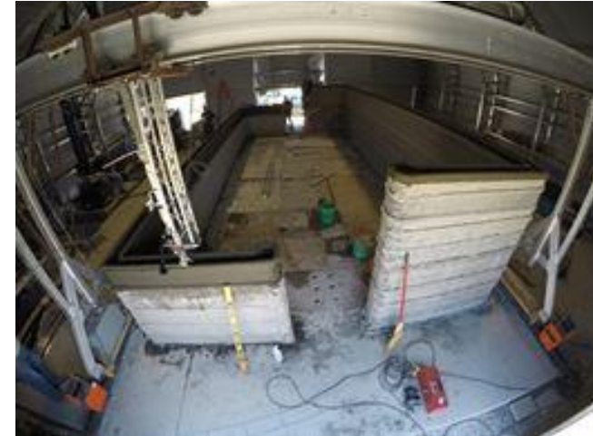
NASA Additive Construction for Mobile Emplacement (ACME) / ACES US Army Corps of Engineers
