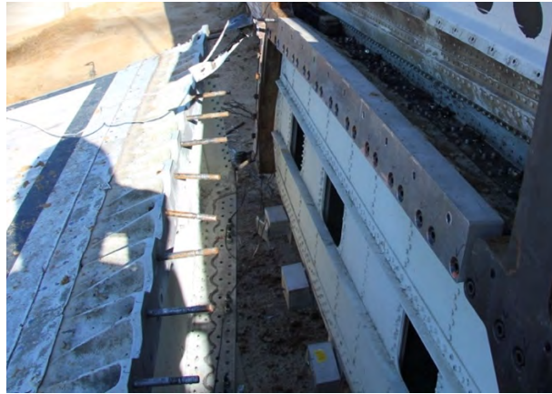
(b) Photo of port wing separation.
