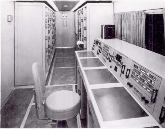
FIGURE 2-16. System test station operator's console.
