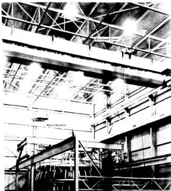
FIGURE 3.—Head handler and overhead crane.
