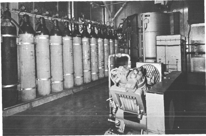
Fig. 17 — Installation for retrieving helium.
