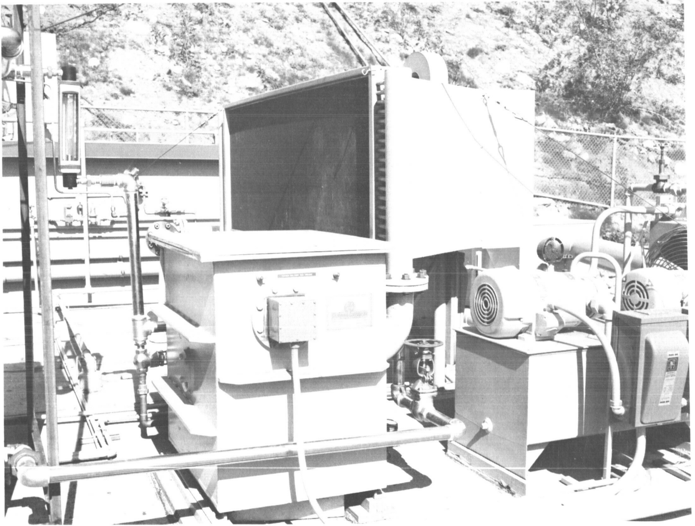
Fig. 49. Argon heat exchanger and blower housing
