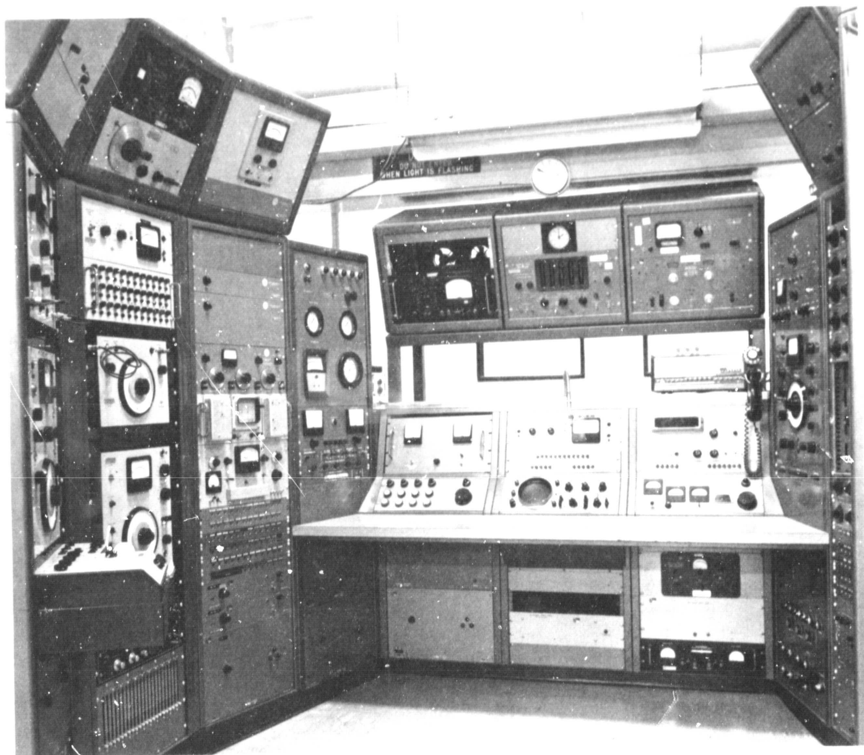
Fig. 7. Monitor and control console
