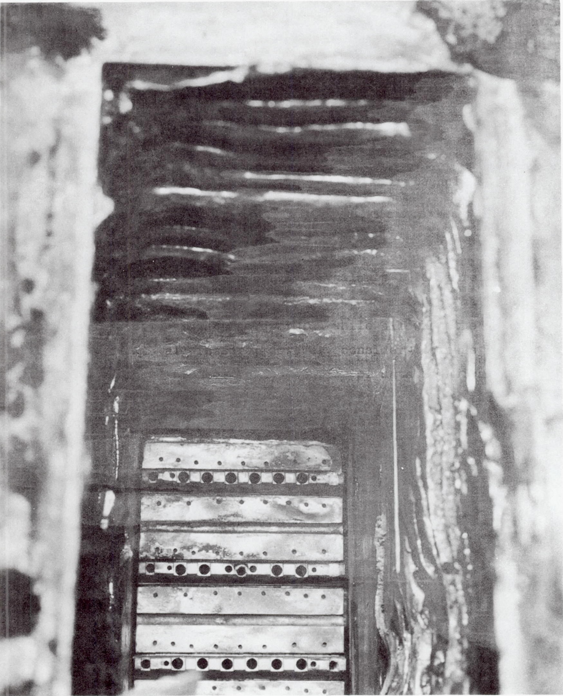
Figure A1-2. Eroded Upper Combustion Chamber - Right Hand Side
