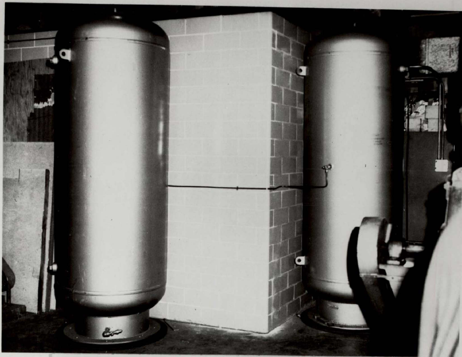
INSTALLATION OF CLOSED CYCLE SUPERFLUID LIQUID HELIUM REFRIGERATOR WITH COLLINS/ADL HEAT EXCHANGER AND ACCESSORIES FOR SUPERCONDUCTING HIGH VOLTAGE CRYO ELECTRON MICROSCOPE 1969
