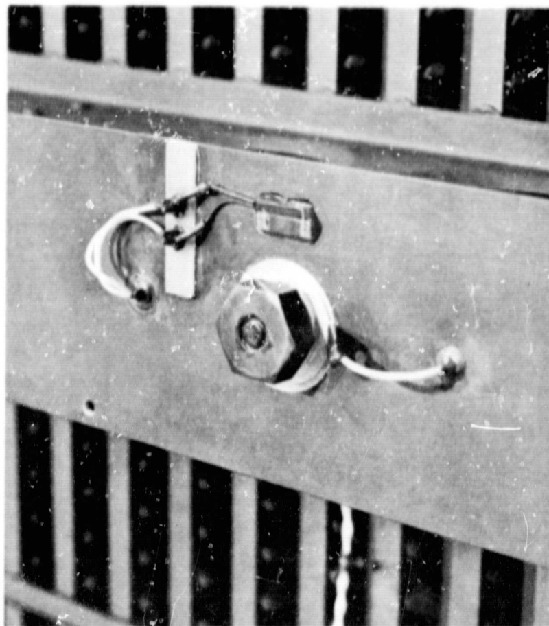
Fig. 6. Closeup of typical temperature transducer installation
