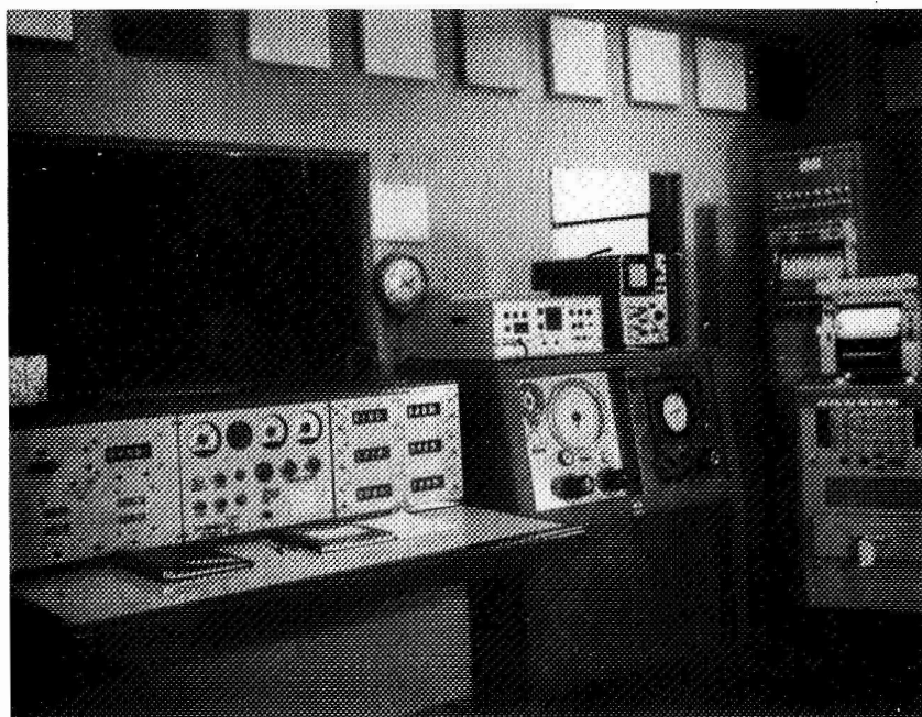
FIG. 4. Control Panel and Recorder
