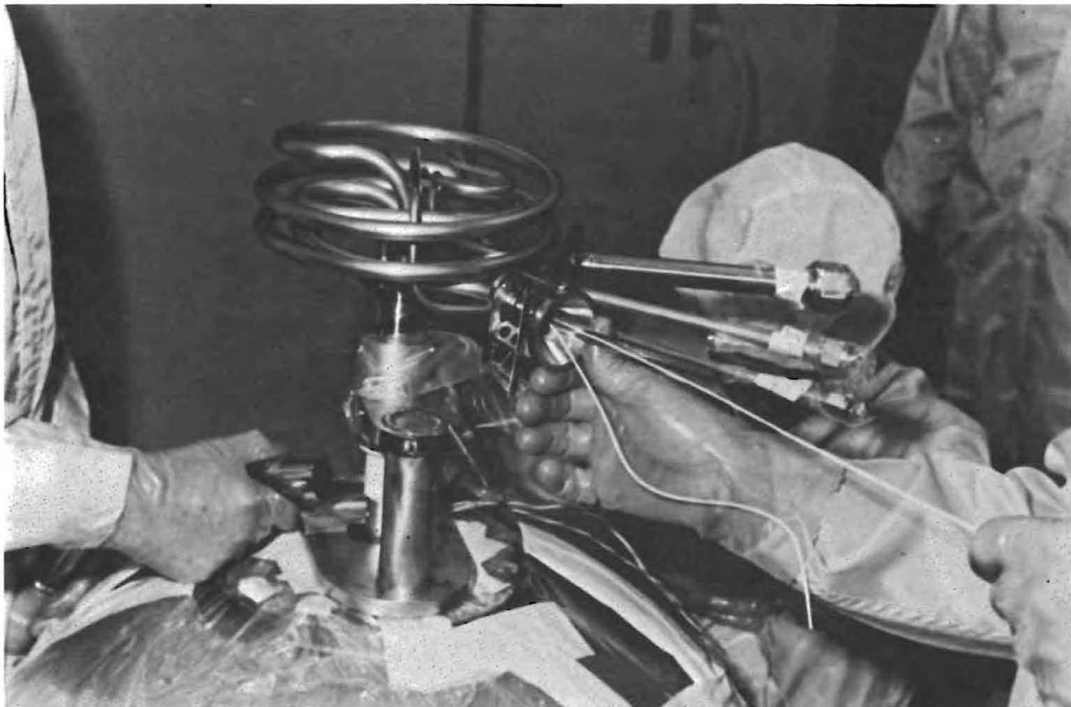
Figure C4-41.- Pull wire used to route heater and fan motor leads into upper coil assembly.
