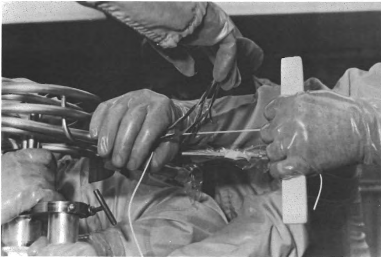
Figure C4-40.- Pulling first bundle of heater and fan motor leads into upper coil assembly.
