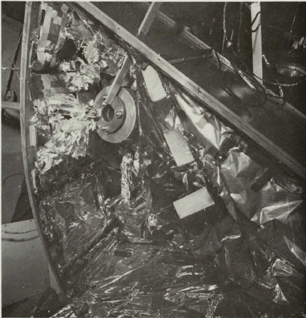
Figure B. 52-3.- Damage to multilayer insulation by impingement of oxygen stream.
