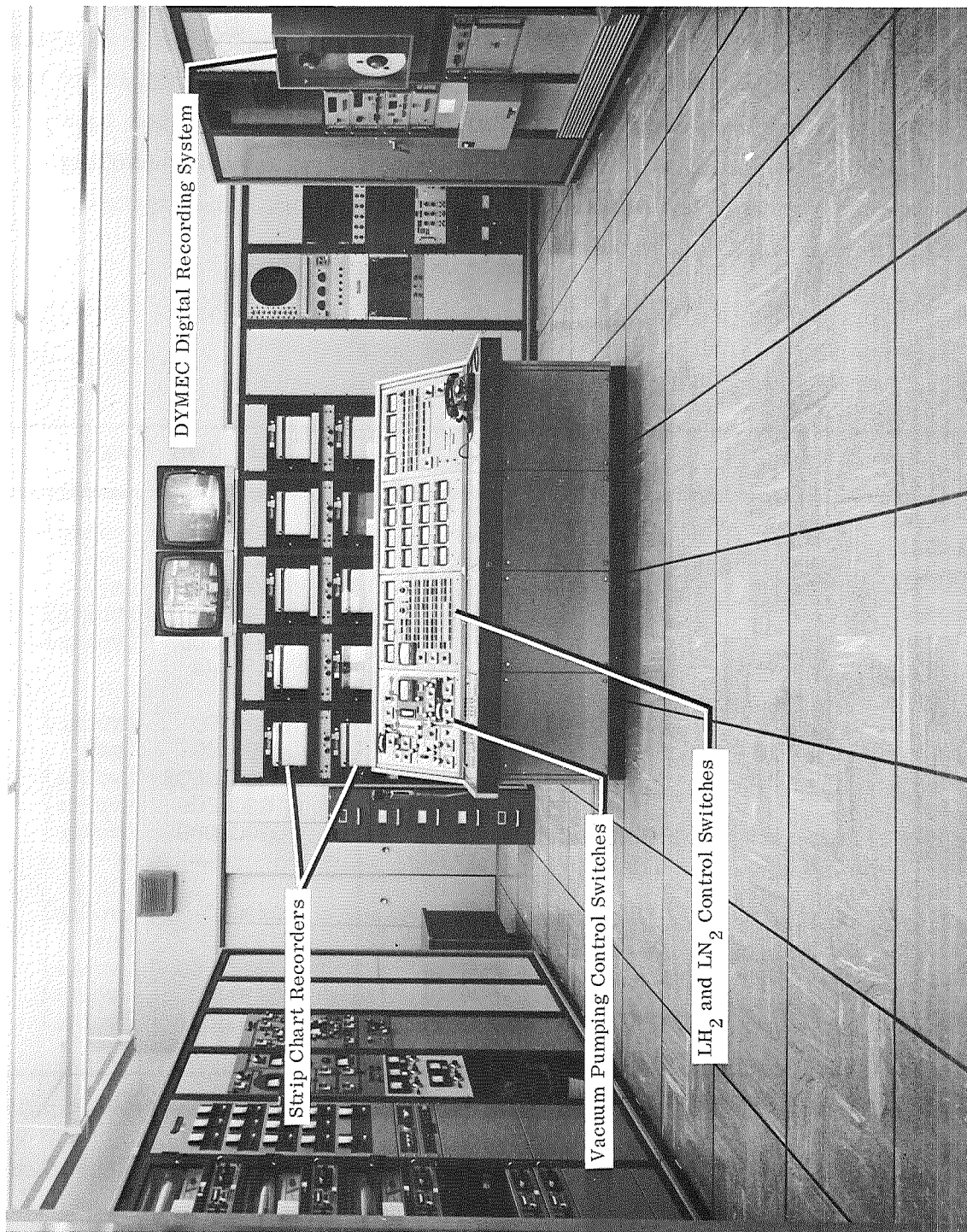
Fig. 3-11 Interior View of the Control and Instrumentation Building
