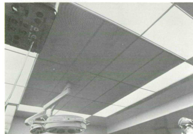
Clean air distributes through perforated epoxy-coated panels with a maximum linear velocity of 1.27 ft./sec. A service column is in the upper left corner.
