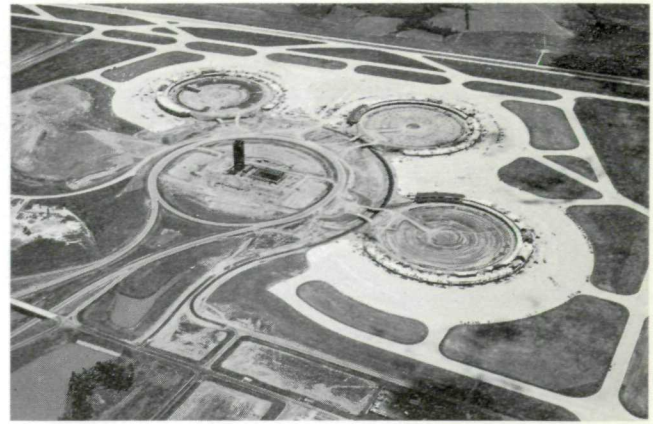
Recent aerial view of construction at KCI illustrates the three terminals with exterior aprons and central parking. The entrance road encircles the Control Tower and Airport Operations and Management Building.
