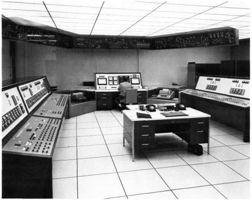
FIGURE 4.105 Lone Star Cement Control Center, Greencastle. [Photograph courtesy of Leeds & Northrup Company.]
