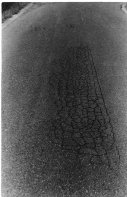
Figure 5—Alligator Cracking in Rolla Glasphalt Road
