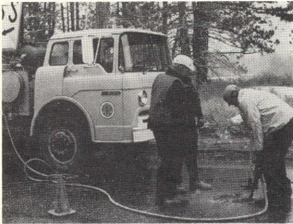
These men are making a pothole.
