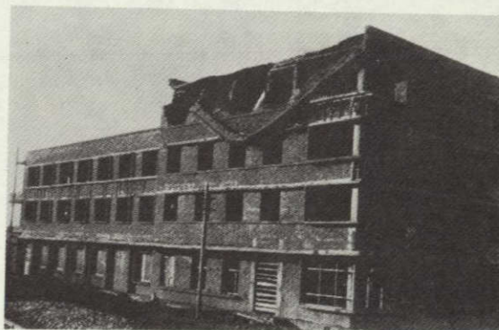
Photo 4: The top portion of a service building east of Panshanching railway, Panchin district, (unfinished) was destroyed by the tremor. Cracks appeared in many places. (Mag 7 area)
