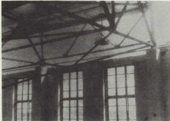
Figure 17: Damage in horizontal support
