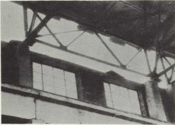
Figure 15: Upper part of this vertical wall collapsed
