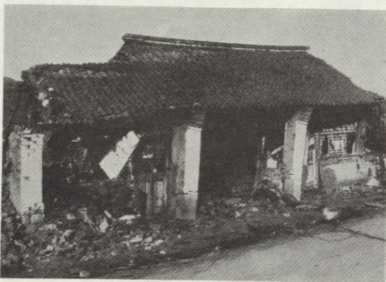
Photo 1: Haicheng District Punkao People's Commune. Most houses in this area collapsed. Most walls fell to the west. The front pillars of this brick house leaned east. Walls separating rooms all collapsed. The machine factory stood to the right of the house, but collapsed after the earthquake. (Mag 9 area)
