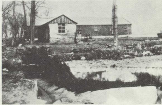
Photo 16: Cracks appearing in the earth in Tienchiang-Tai paper mill in Panchin district were 3.2m wide according to a report. When the photo was taken on 12 Feb., the width was 2.4m and the crack ran northeast ( 50^{\circ} ) with a visible depth (to water surface) of 1.5m, left displacement 14.5cm. (Mag 8 area)
