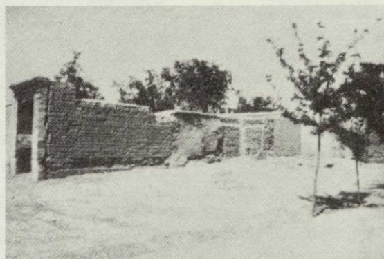
Plate 3: Damaged areas in Yingtai earthquake of 1966 (above)
