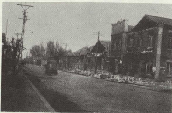
Photo 3: The bath house in Taishihchiao, Yingkao Prefecture. Top portion of the end walls fell with the tremor. (Mag 9 area)
