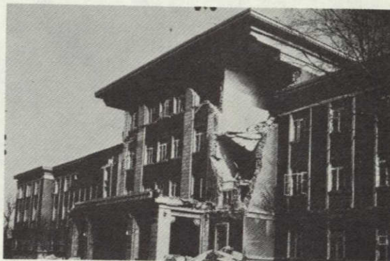
Photo 2: The front of this Haicheng Guest House partially fell after the quake. Cracks appeared in many places. (Mag 9 area)
