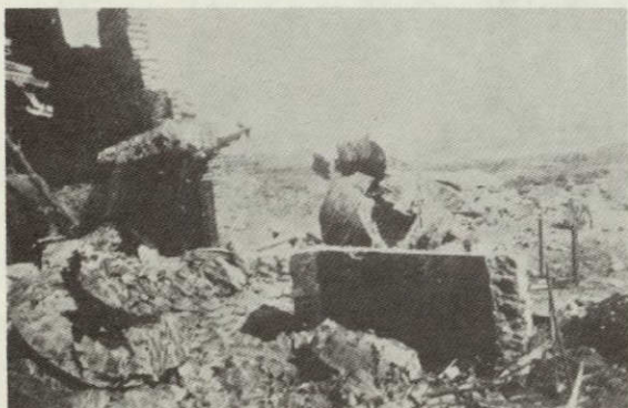
Photo 9: A cylindrical brick chimney of a paper mill in Yingkao Prefecture, operated by Kaoken People's Commune - 30m high, base diam. 1.7m, top diameter 1m, 70cm thick - fell in many pieces. The top half fell southwest, smashing the boiler room. Base portion fell toward the north. (Mag 8 area)
