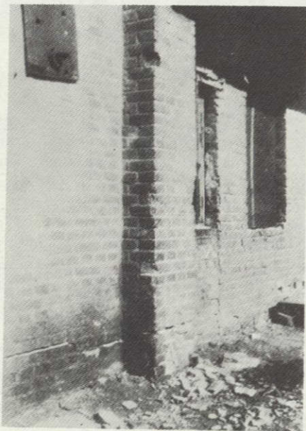
Figure 9: Damage in the lower part of a factory building with brick pillars
