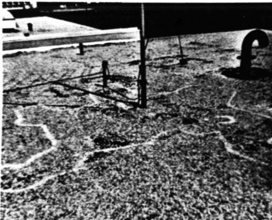
FIGURE 13. AN ANTENNA INSTALLATION OF BUILDING 162, VINT HILL FARMS STATION. AREA OUTLINED IS UNDERLAIN BY WET INSULATION.
