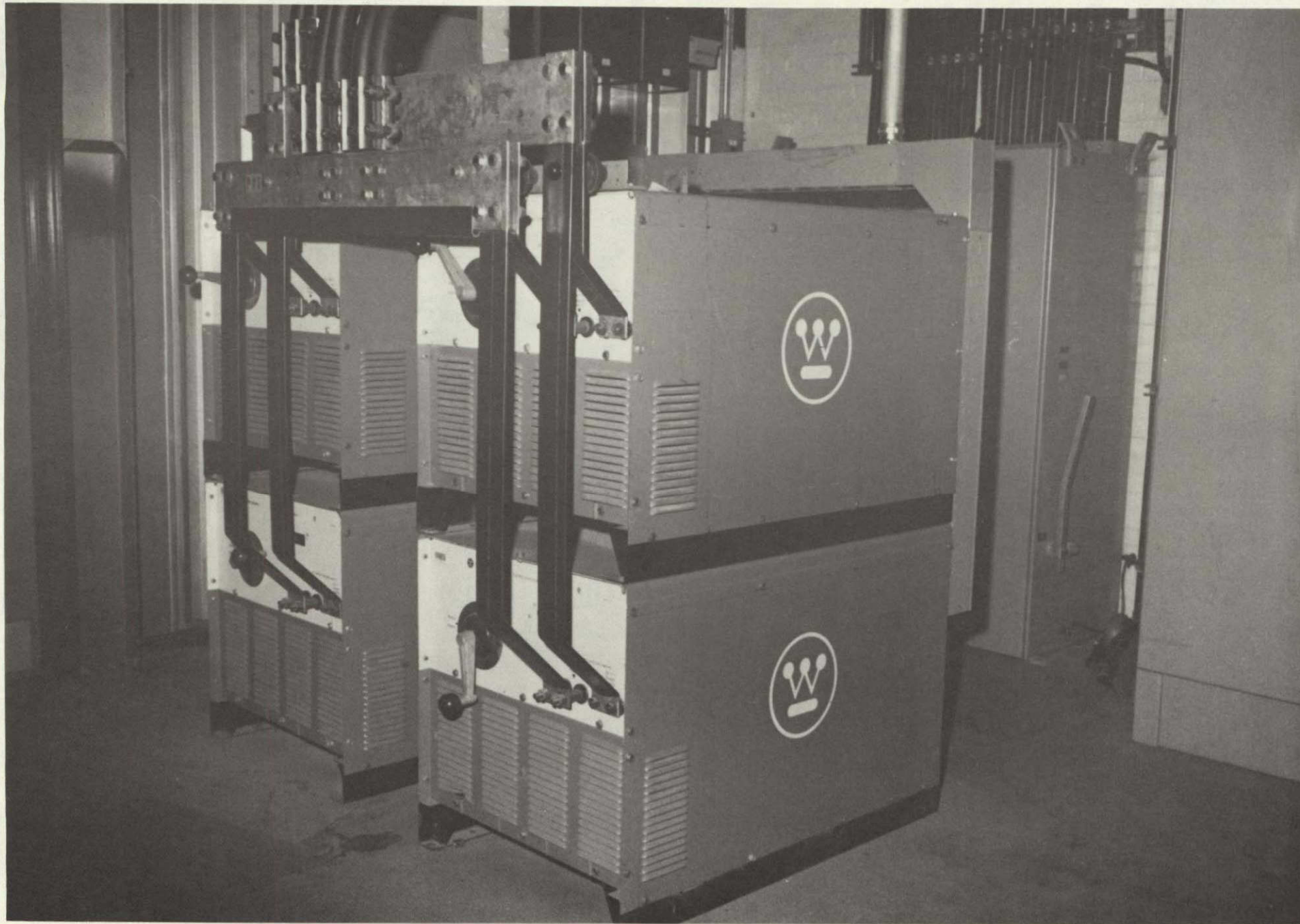
Figure 3.20 - Photograph Of The dc Welder Units Which Supply Arc Heater Field Coil Power
