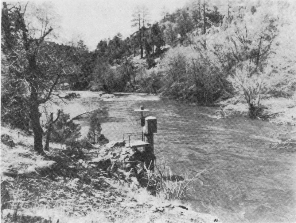
Figure 31. Black River near Point of Pines gaging station equipped with a Landsat data-collection platform.
