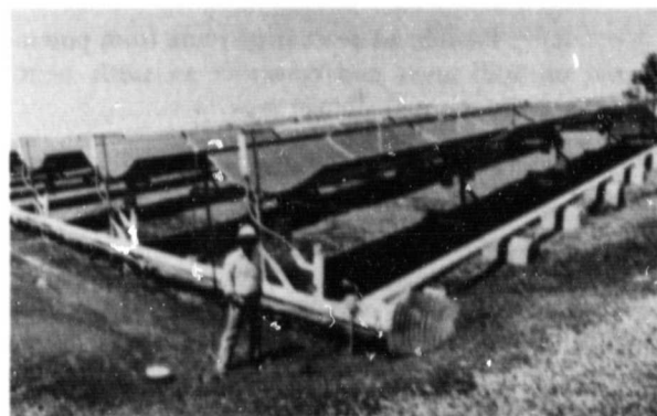
Figure 4-17. Collector Field at Dow Chemical Plant
