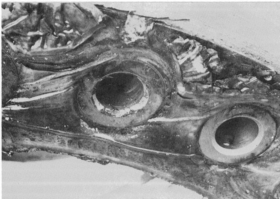
(b) Corrosion of face of spool piece.
