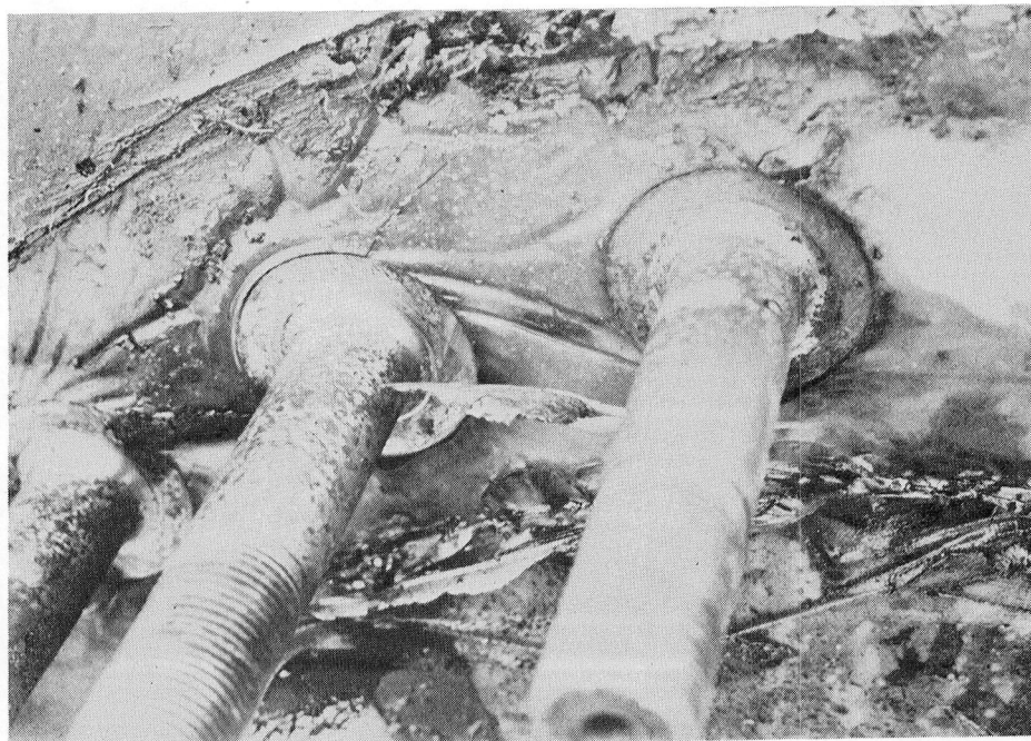
(b) Closeup of general corrosion.
