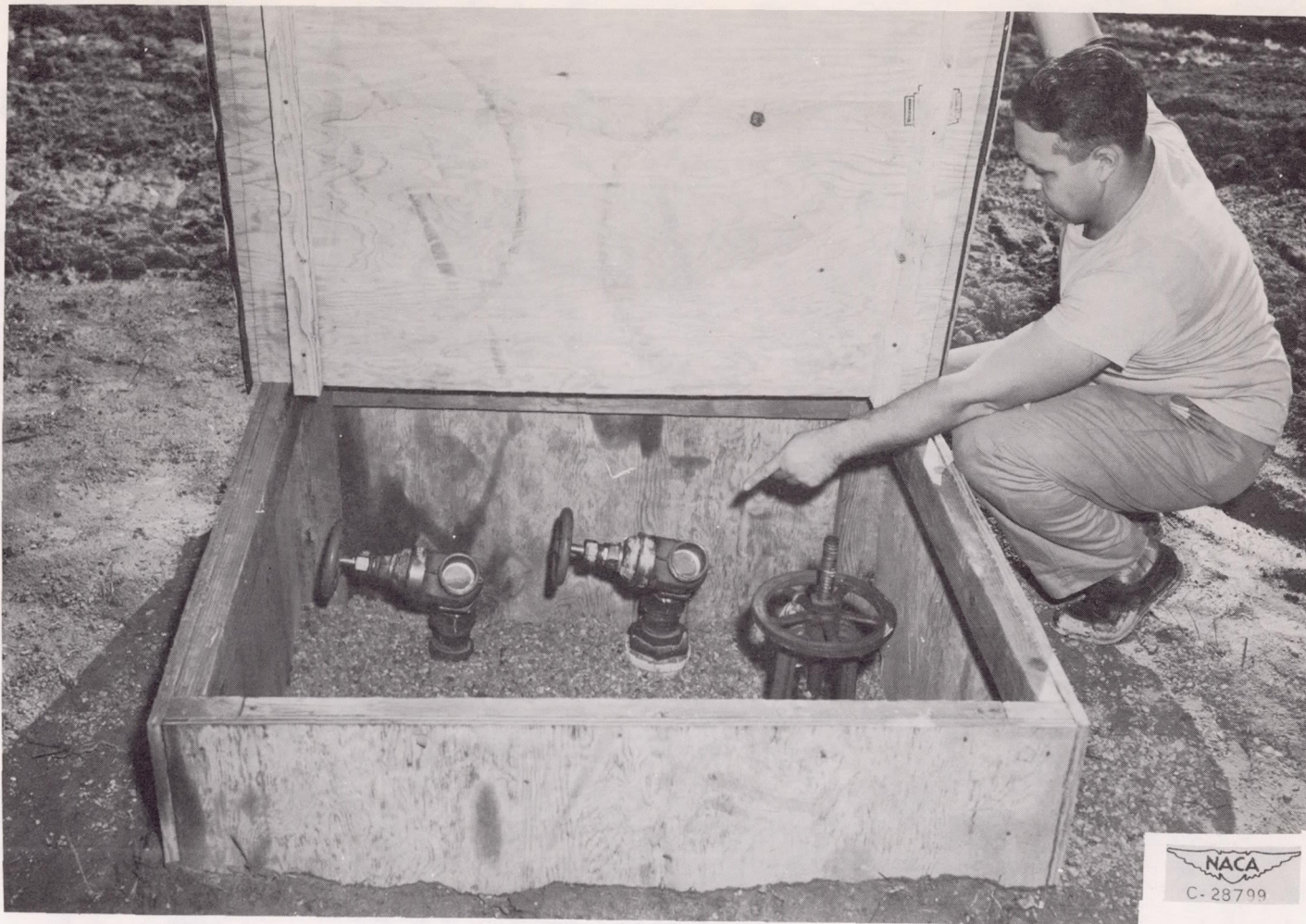
Figure 19. - Fire protection outlet located on each side of crash area.
