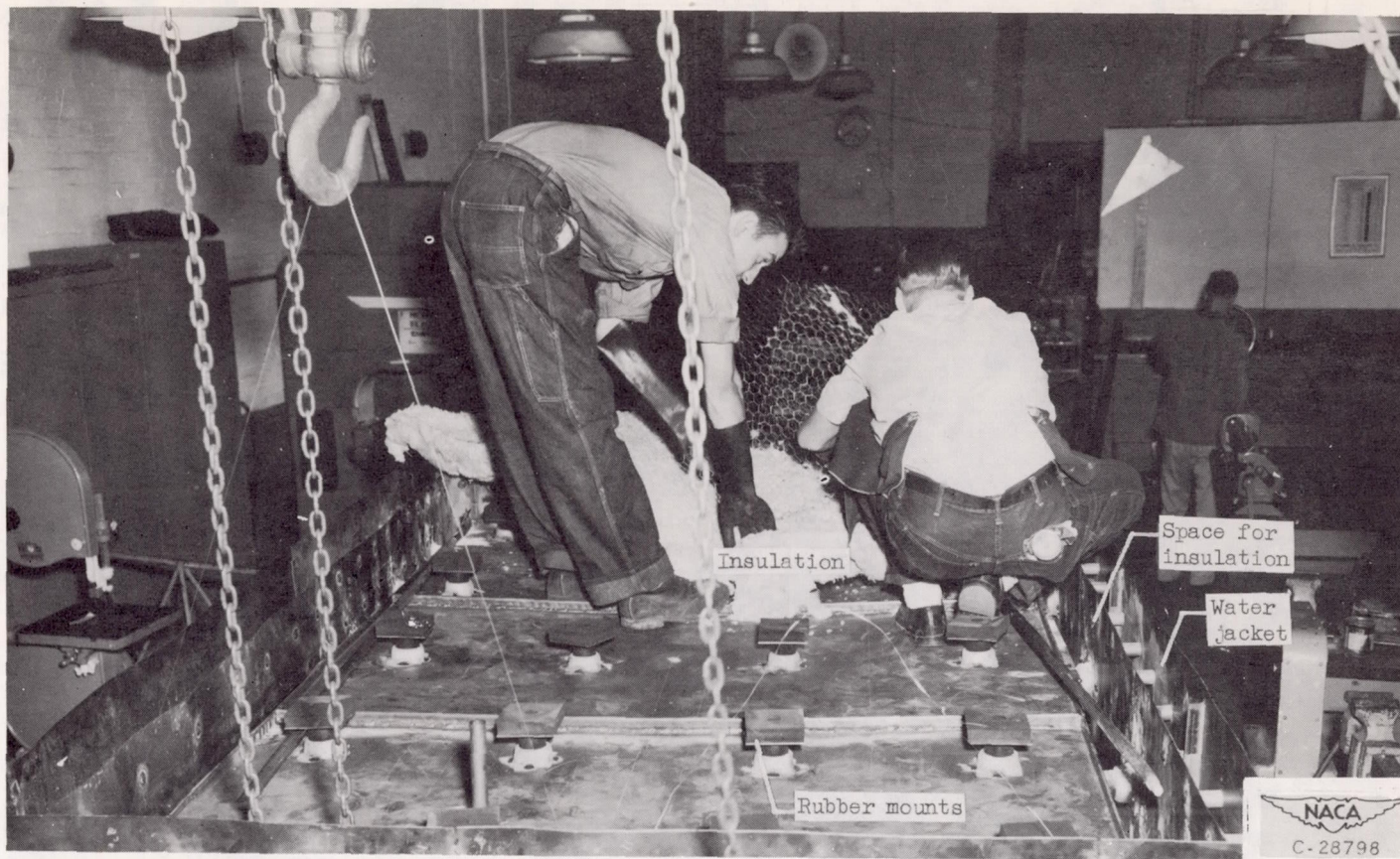
Figure 21. - Three-quarter top view showing construction of fireproof instrument box before top was installed.
