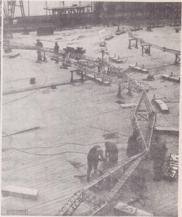
Figure 20.- LZ127-Main ring on the floor. The rings are completely finished on the floor and are erected by the aid of stiff assembly frames.
